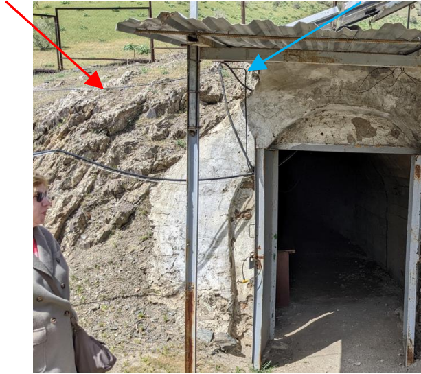
Figure 41. Fiber optic cable entering the tunnel. The red arrow shows the line. The blue arrow shows an undesirable sharp bend in the cable.
