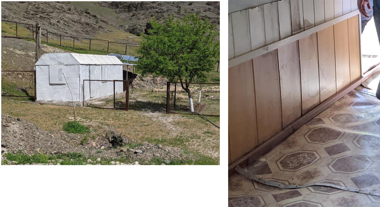
Figure 40. Left – Overview of the wagon building. The tunnel entrance is behind the wagon and under the solar panels. Right - Evidence of water ingress and rot in the collapsing floor of the wagon.
