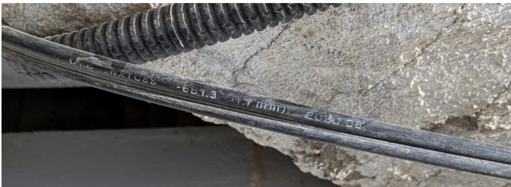
Figure 42. Close-up of the fiber cable with identification markings. The cable appears to read 'CPC NXTCS -6B1.3 (1.7 mm) 2020.08'
