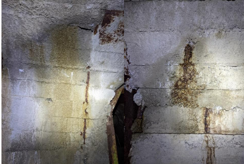
Figure 48. Water seeps on the wall to either side of the entrance to pier 2.
