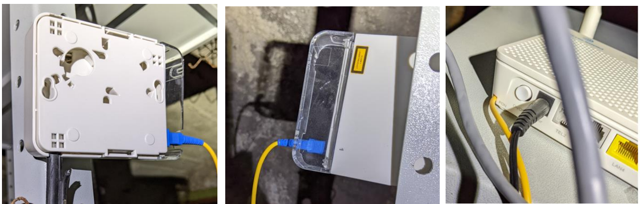
Figure 43. Fiber cable with junction box (left and Center) and switch (right). Cable is incoming at the bottom left of the image at right.
