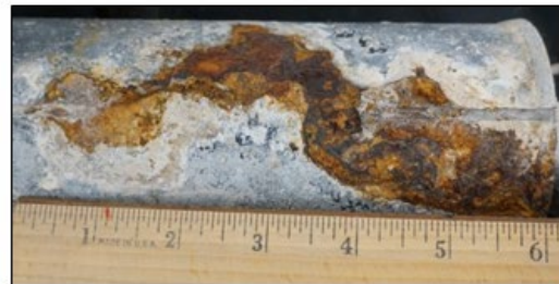
(b) Corrosion of pipe sleeve
