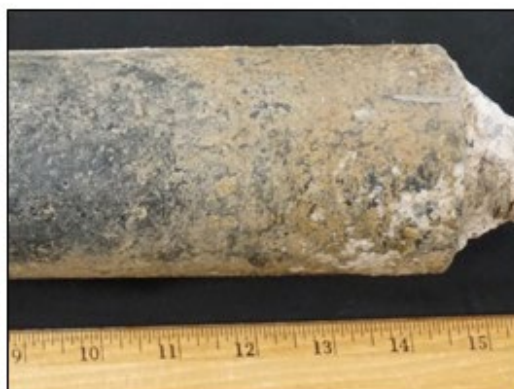
(f) Top of the pipe sleeve with discoloration
