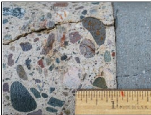
(a) Cracking terminating in cap
