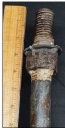
(b) Cracking and deterioration at the surface
