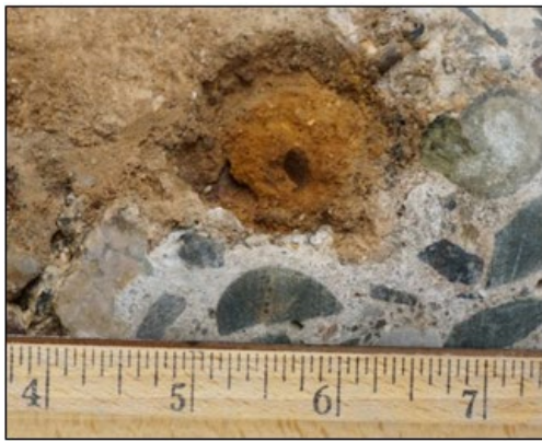
(a) Corrosions and deterioration of concrete
