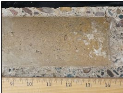
(e) Concrete after extraction of pipe sleeve showing discoloration at the top
