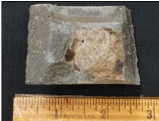
(c) Cracking around the bolt with corrosion
