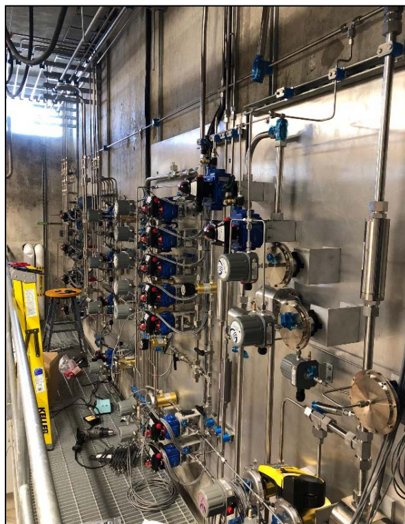
Figure 22: HPL Test Cell 4 facility plumbing which will be used for the high-pressure plasma-assisted burner.
