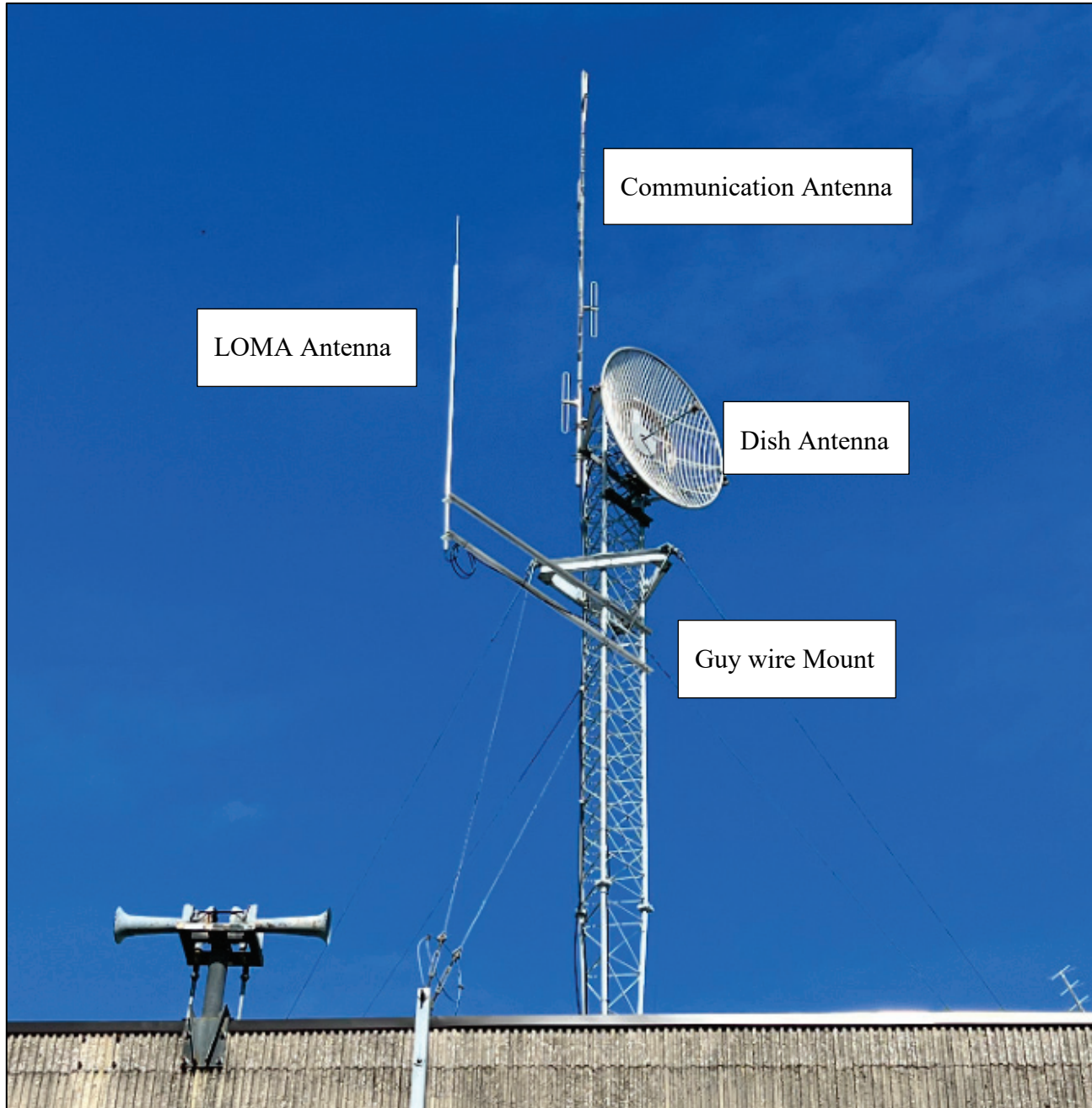
Figure 4. The new LOMA antenna location on the left side of the tower.
