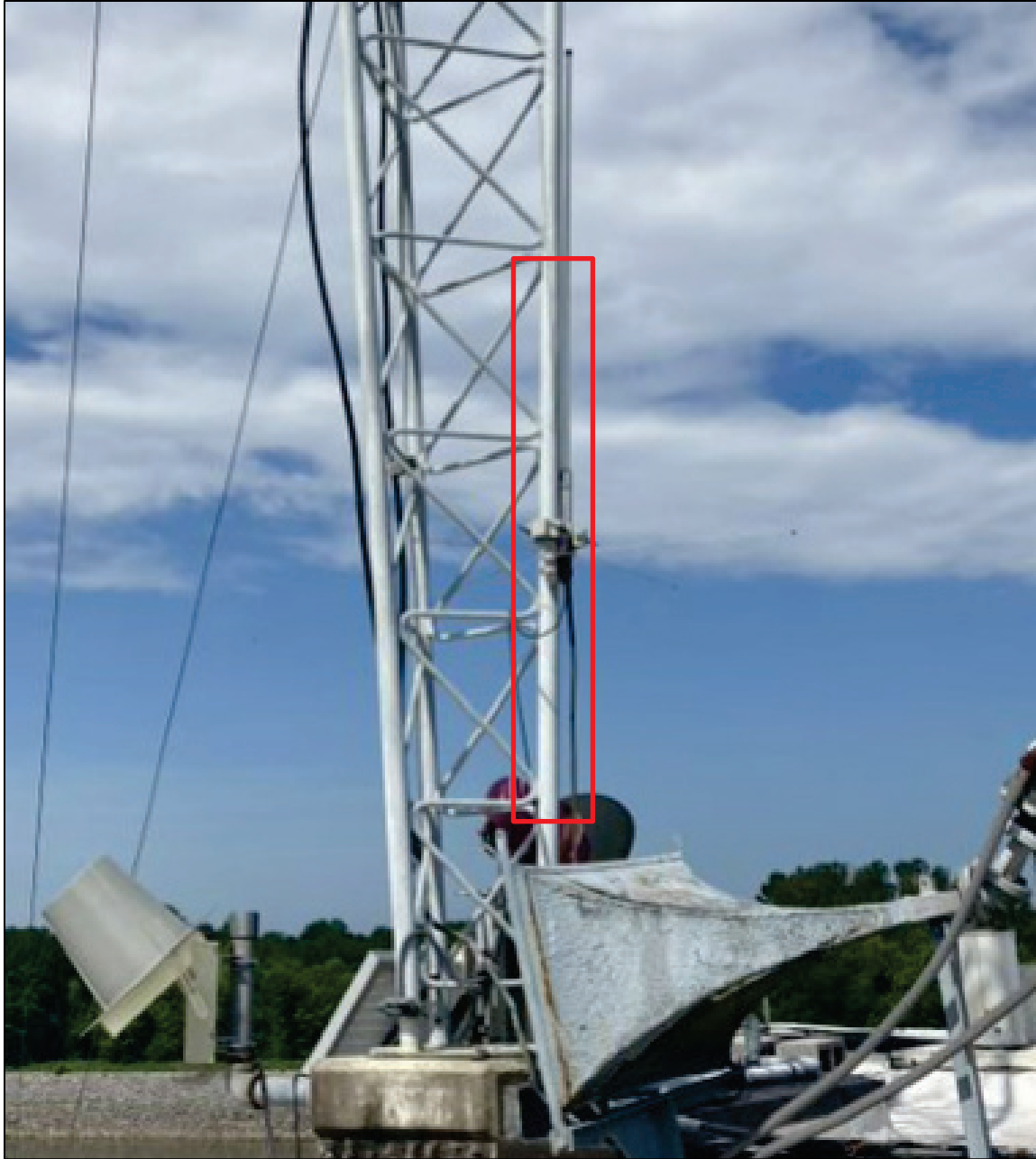
Figure 2. Original LOMA antenna (inside red box ) mounted just above the roof alongside the base of the tower.
