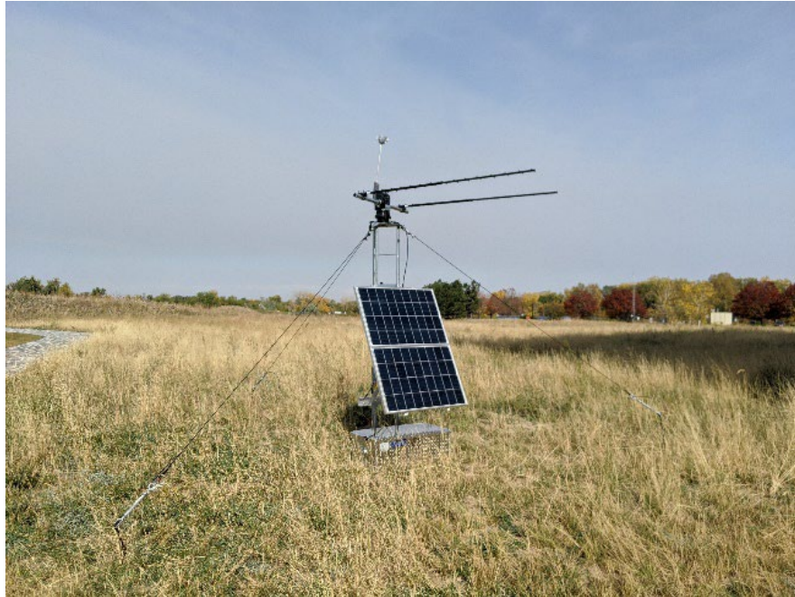
Figure 14 Installed Distributed Ground Receiving Station (DGRS). These were used for the majority of the flights conducted in the post-COVID shutdown period.
