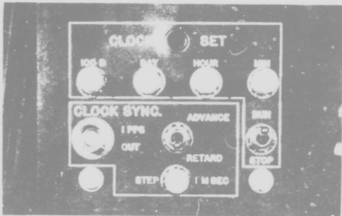
(a) Clock controls on front panel of control unit
