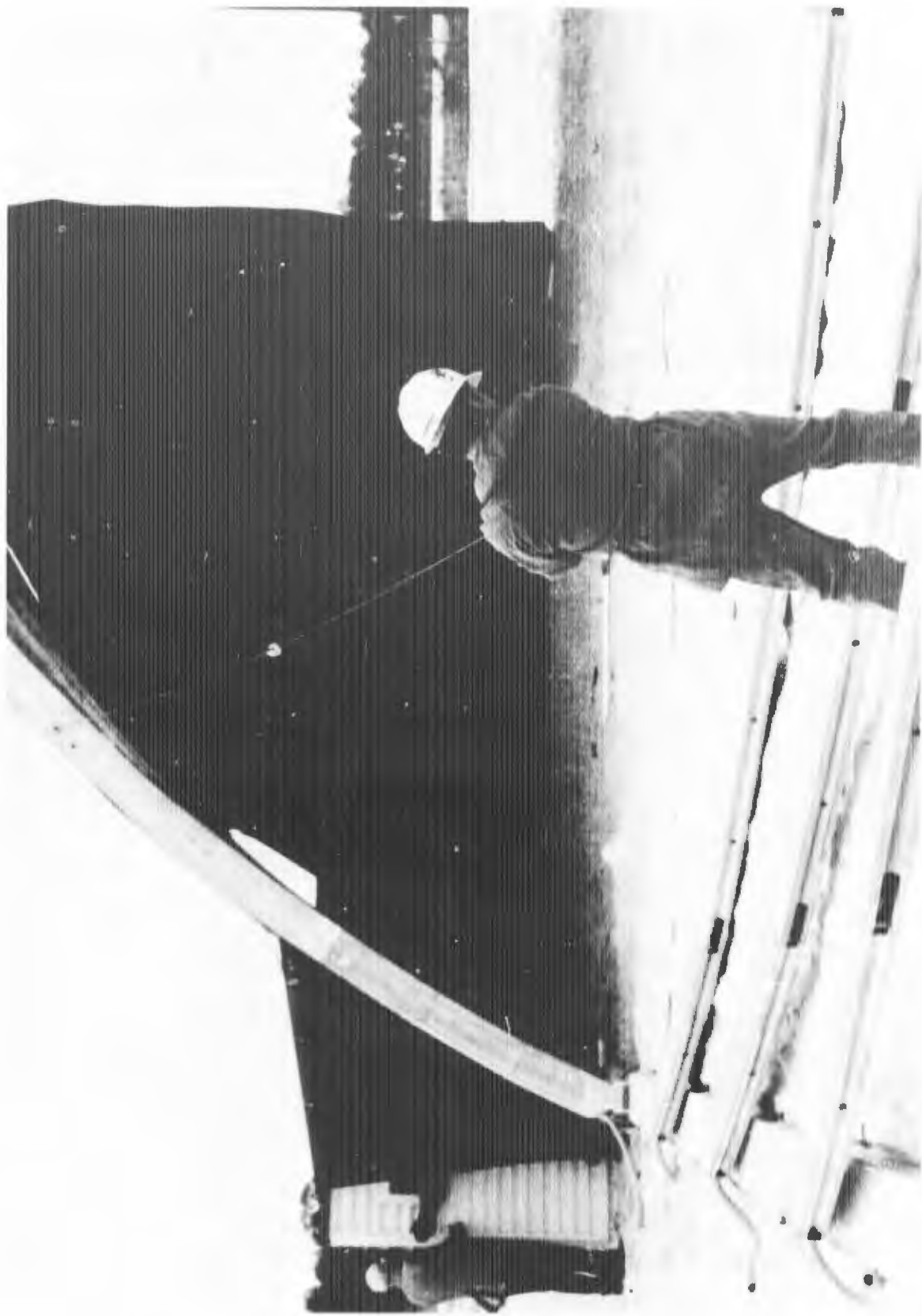
Figure 33 Cable Being Attached to Sixth Arch of Side Entry System in Place
