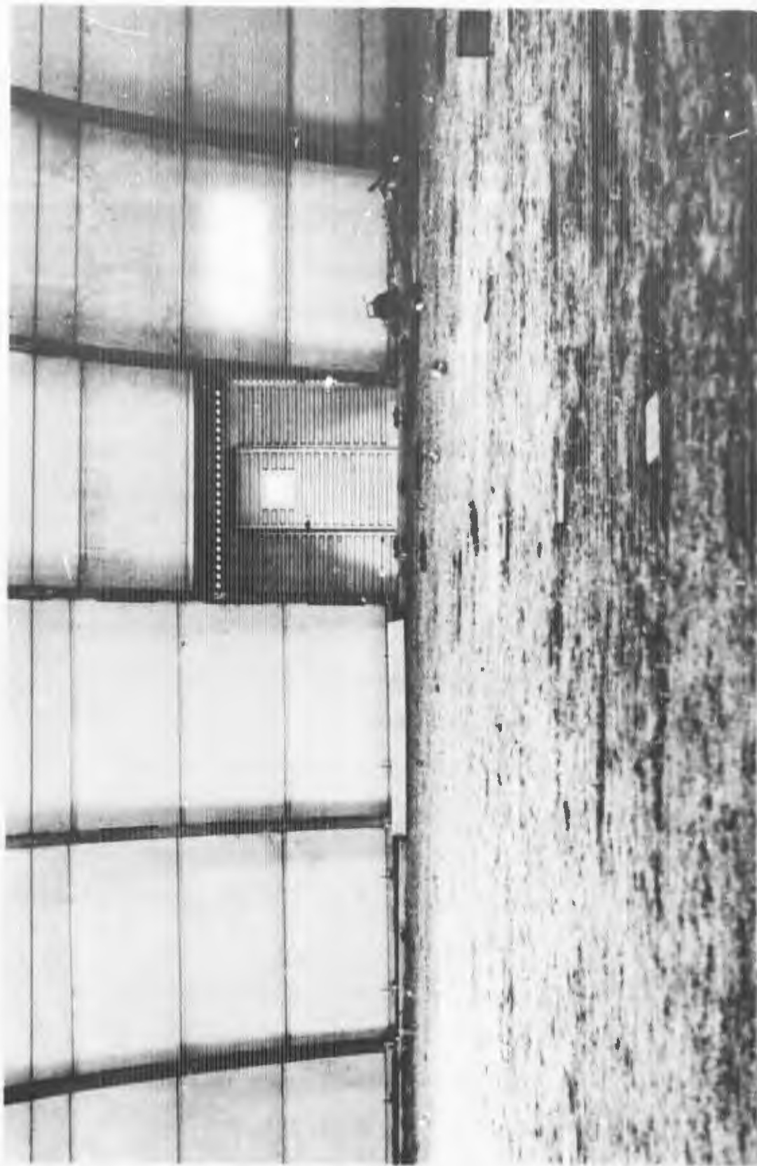
Figure 86 Overall View of Data Collection Points and Deflection Across the Arch Beams
