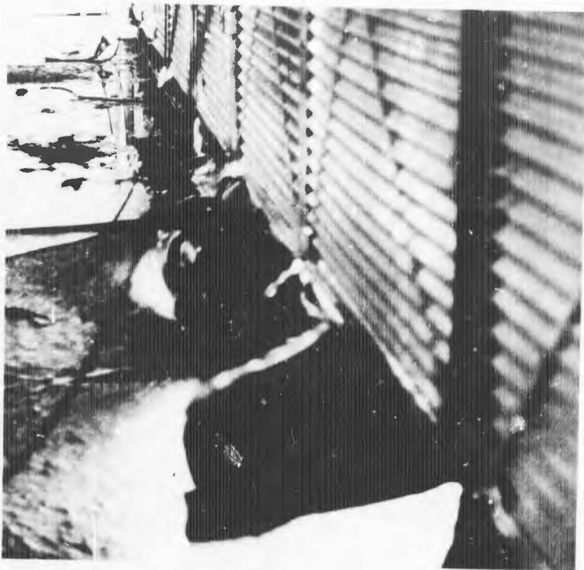
Figure 95 Water Leakage Under Metal Door and Ground Skirt Being Blown Inward
