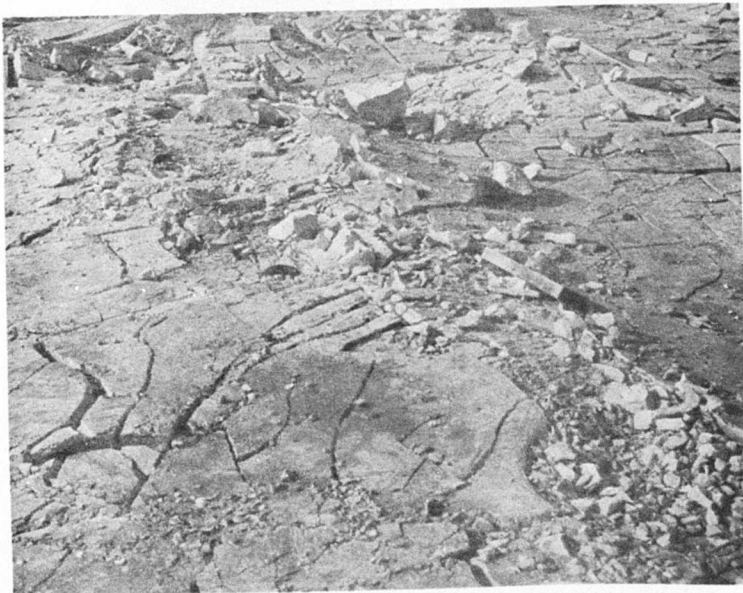
Figure 93. Test 2-1, No Load Deterioration of Reg-set Surface
