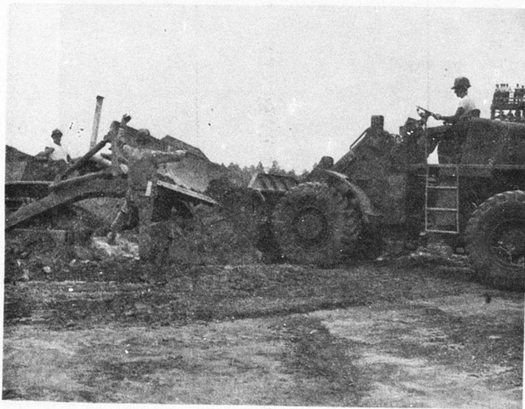
Figure 18. Test 1-1, TD 20 Inside Crater Aiding AC 645 in Removing Large Upheaved Pavement Sections
