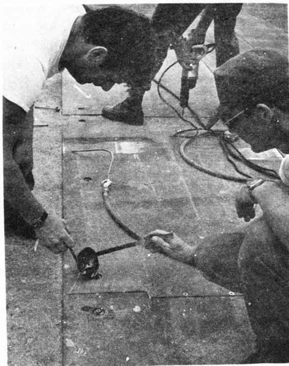
Figure 56A. Test 1-2, Molten Lead-Sulphur Ramp Attachment Method of Pouring Lead-Sulphur Compound into Drilled Hole. Bolts and Device Used to Clean Hole are Visible in the Background
