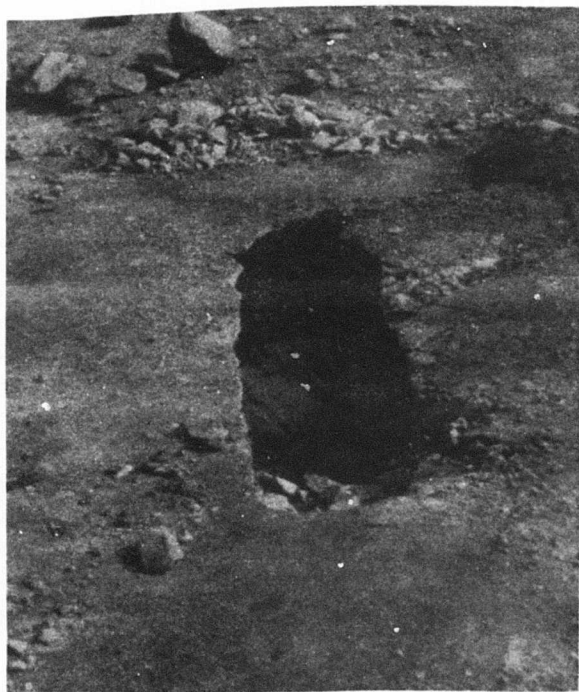
Figure 91. Test 2-1, Punching Failure under Load Cart Wheel
