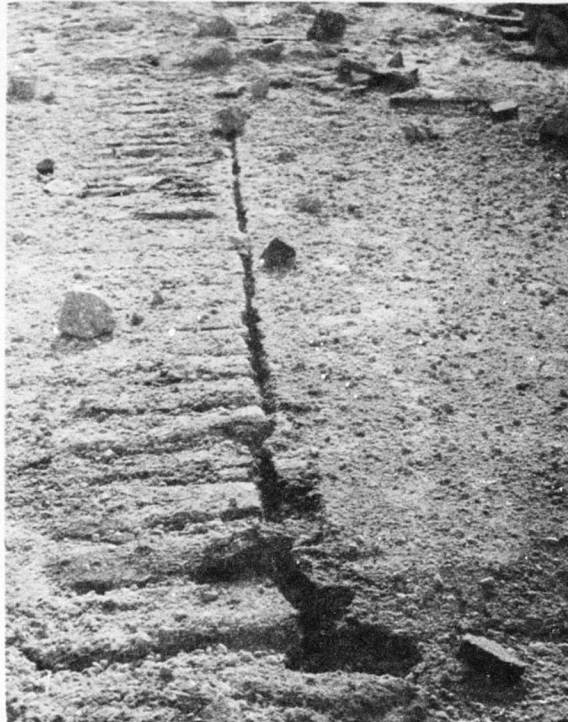
Figure 125. Pavement Cracking Outside Zone of Upheaval, Test 1-2
