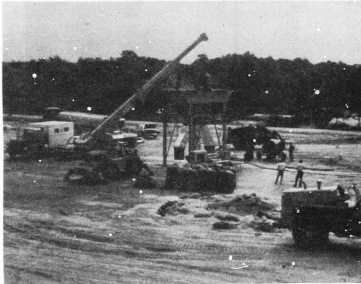
Figure 107. Feeding of Open Bulk Ready Mix Hopper from Rubber Field Containers
