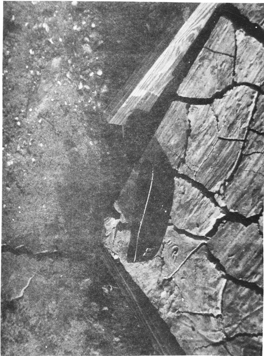
Figure 122. Evidence of Extreme Expansion, Deteriorated Cap, Test 2-1
