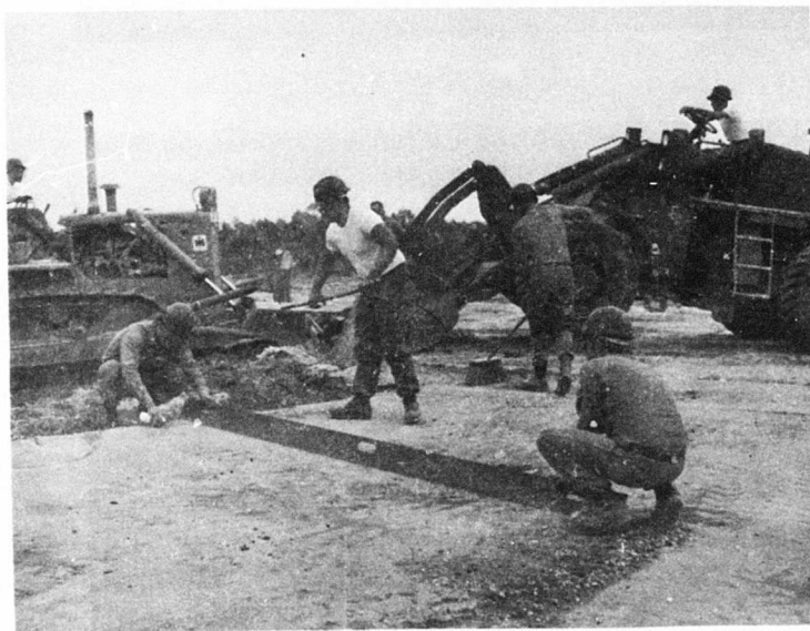
Figure 16. Test 1-1, Identifying Subtly Upheaved Pavement with Specified Straight Edge
