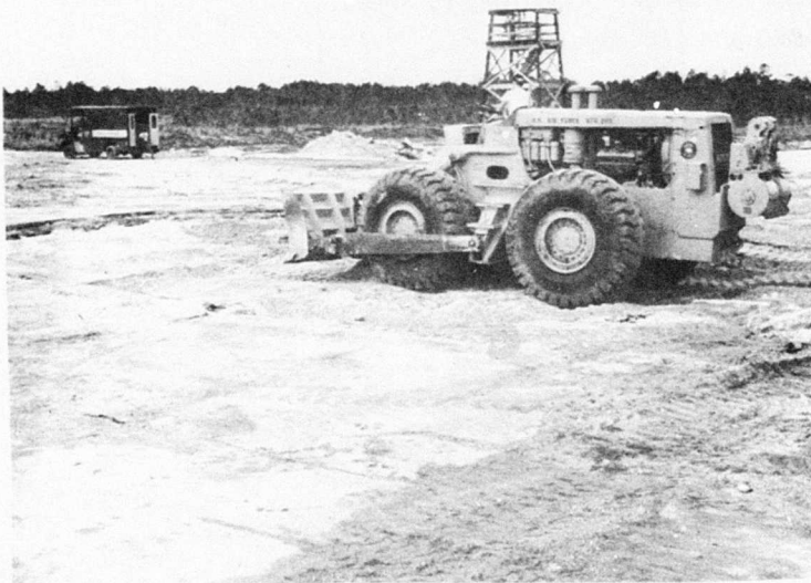
Figure 63. Test 1-3, 280 RT Being Used for Final Compaction of the Debris Subgrade Surface
