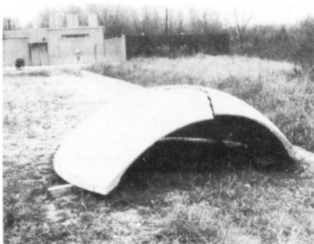
Figure 12. Damage from M67 grenade exploded inside dome.
