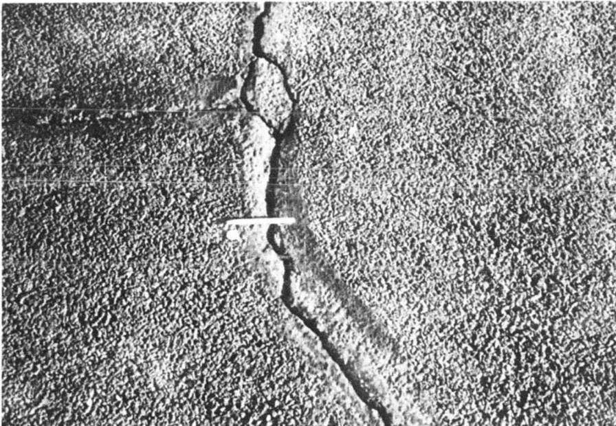
Figure 22. Widened reflected crack (Great Falls)
