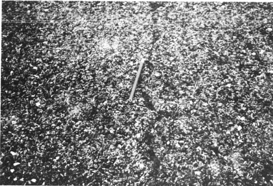
Figure 30. Raveling at reflected crack (Bartlesville)
