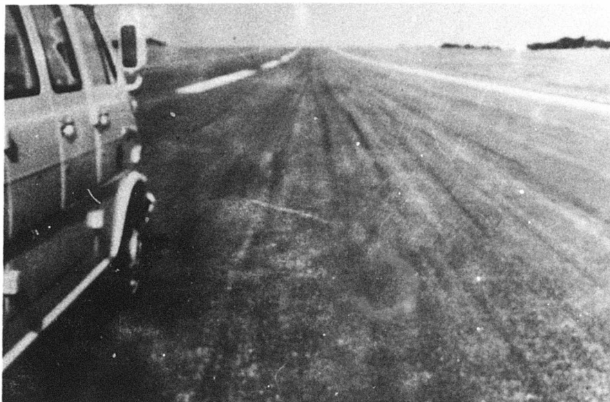
Figure 9. Snow removal damage (Hot Springs)
