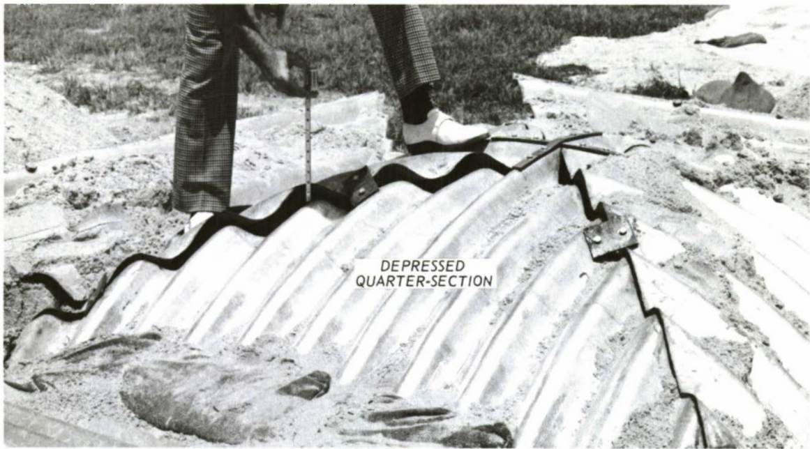
c. Damage to loaded quarter-section of MICS determined after removal of sand cover
