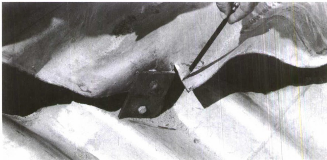
f. Shear failure around one set of connector plates
