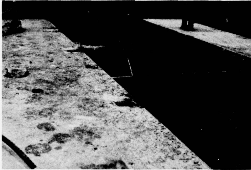
Figure A6. Top view of trashrack showing holes for support bar replacement
