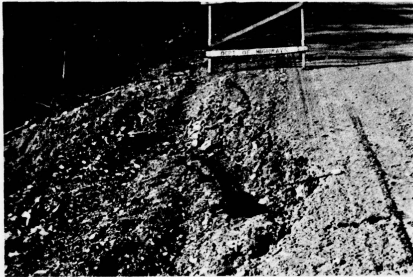
Figure 21. Slope failure along the Elliott Highway
