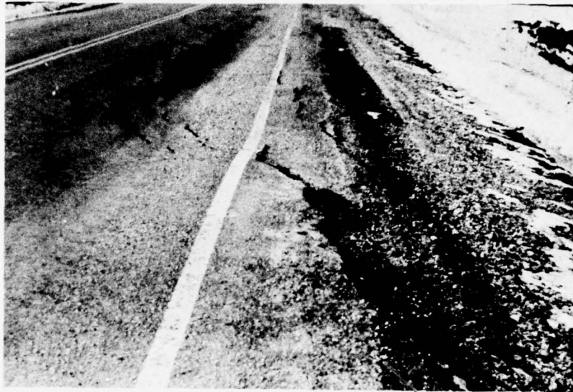
Figure 17. Embankment failure at road shoulder.
