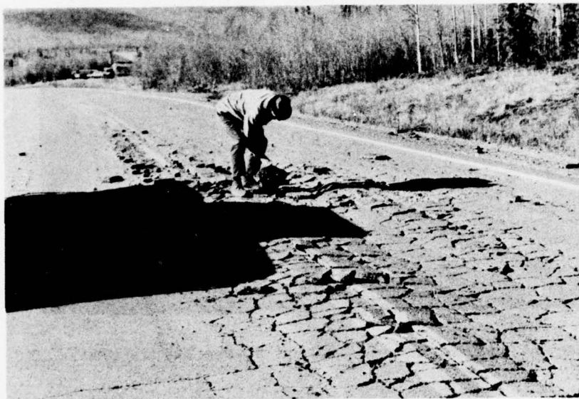
Figure 19. Pavement failure on the Elliott Highway.
