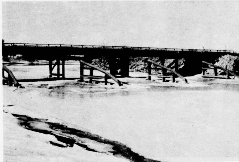
Figure 38. Ice and debris deflectors to protect bridge bents, Engineer Bridge, Fort Wainwright.
