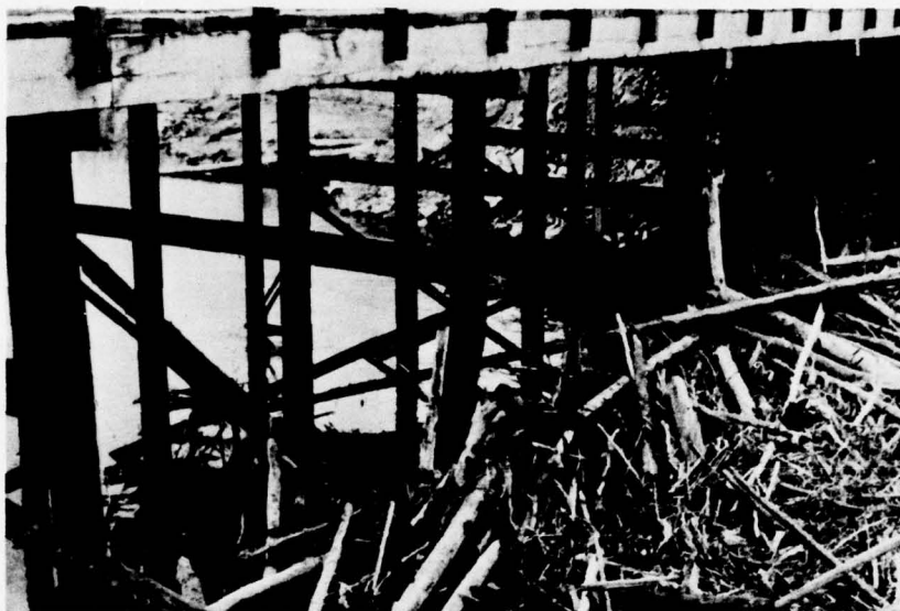
Figure 36. Damage to Hess Creek bridge from ice and debris during high water and ice breakup.
