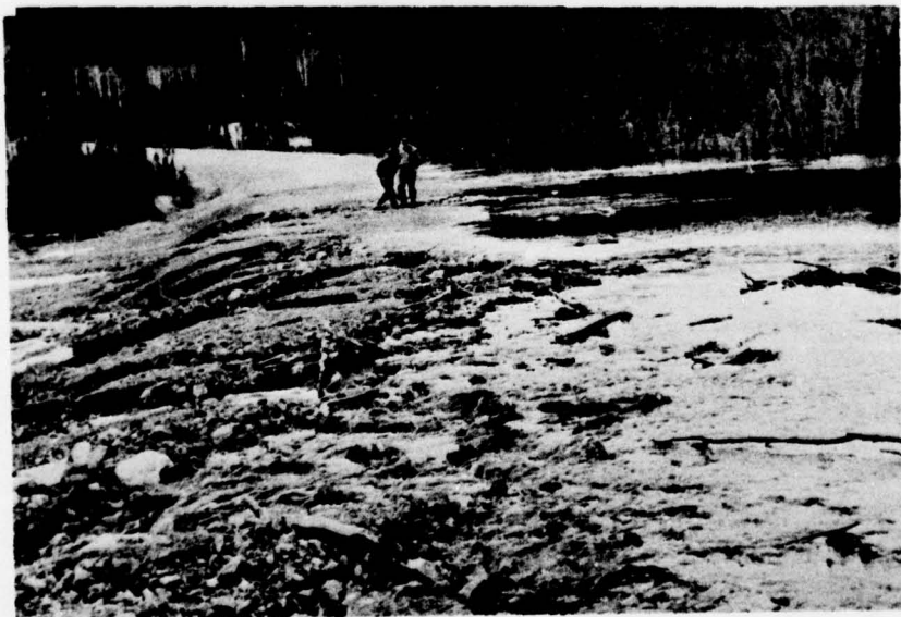
Figure 33. Washout along TAPS road (mile 5.6).
