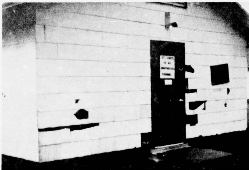
Figure 7. Typical breakages on asbestos cement shingle sidings (Fort Stewart, GA).
