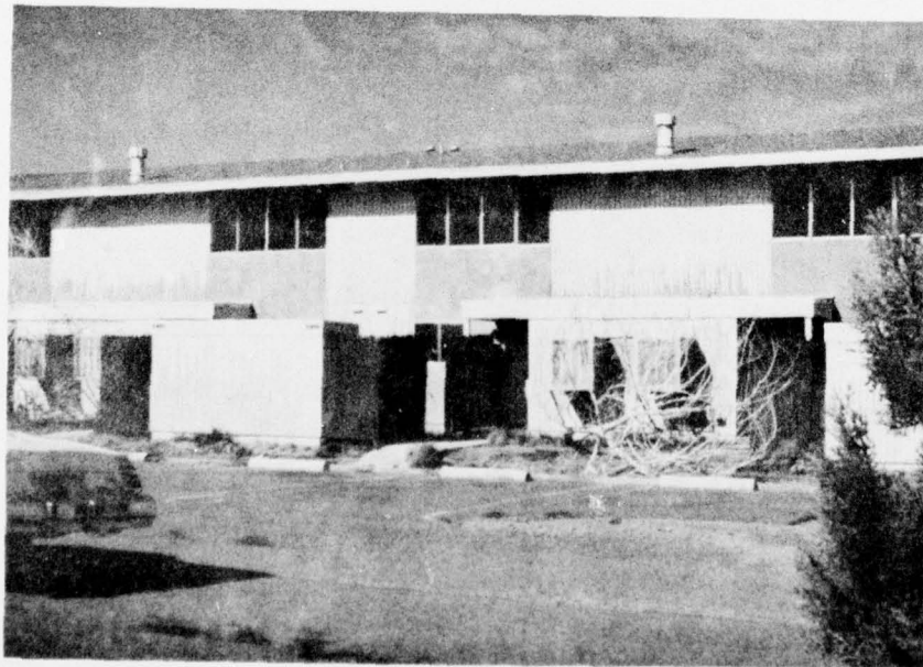
Figure 19. Failure of paints on wood siding due to poor paint-holding quality and sand blasting (Fort Irwin, CA).
