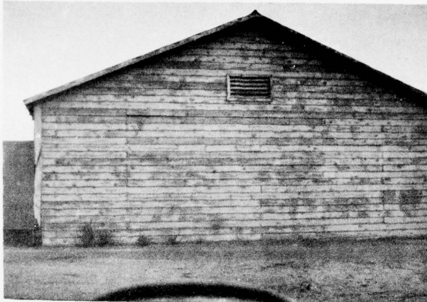
Figure 18. Poor paint-holding quality of wood siding (Fort Irwin, CA).
