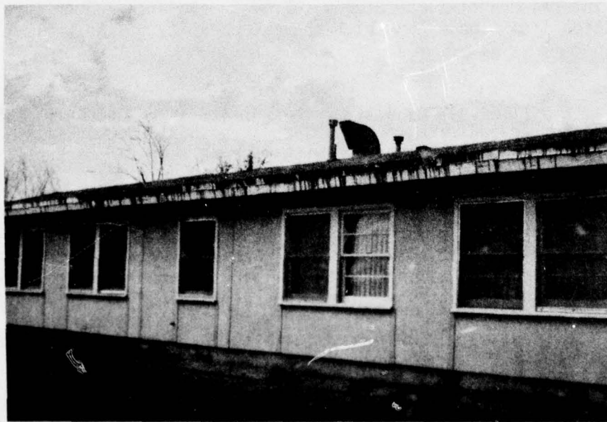
Figure 14. Built-up roofing failure caused by heat. Asbestos cement sheets used for siding are satisfactory (Fort Irwin, CA).
