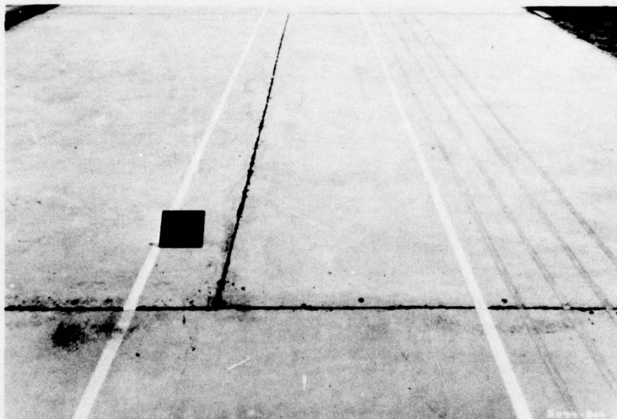
Figure 3-1. Condition of 4-in. fibrous concrete slab on 17-in. cement-treated base before traffic
