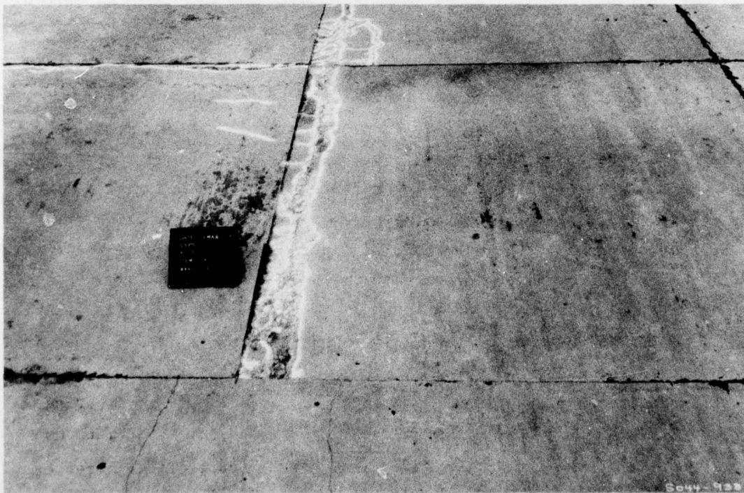
Figure 11-4. Typical joint failure along longitudinal construction joint in rigid subitem 5a
