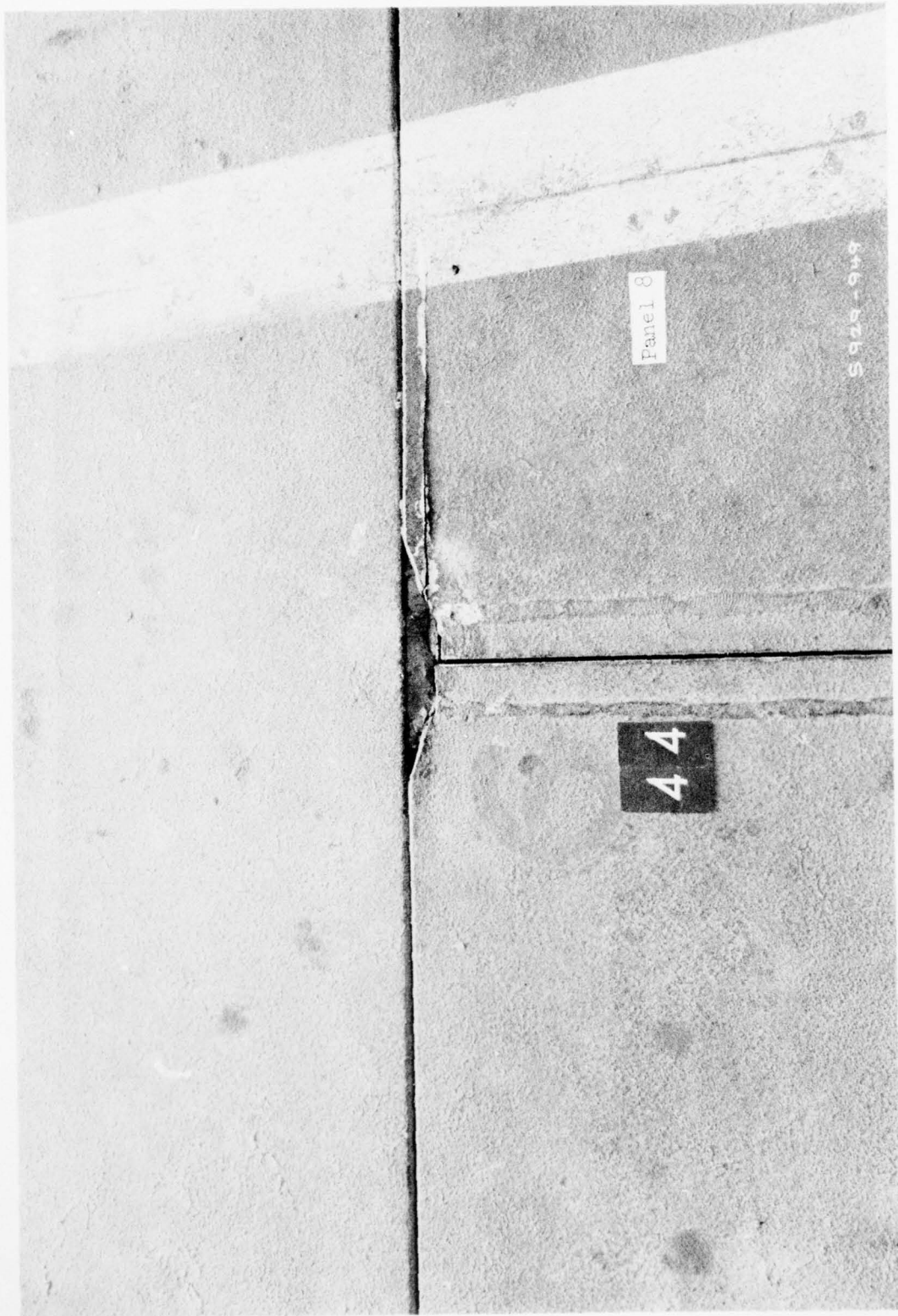
Split in female connector of panel 8 after 210 coverages, Phase 2, subgrade reprocessed
