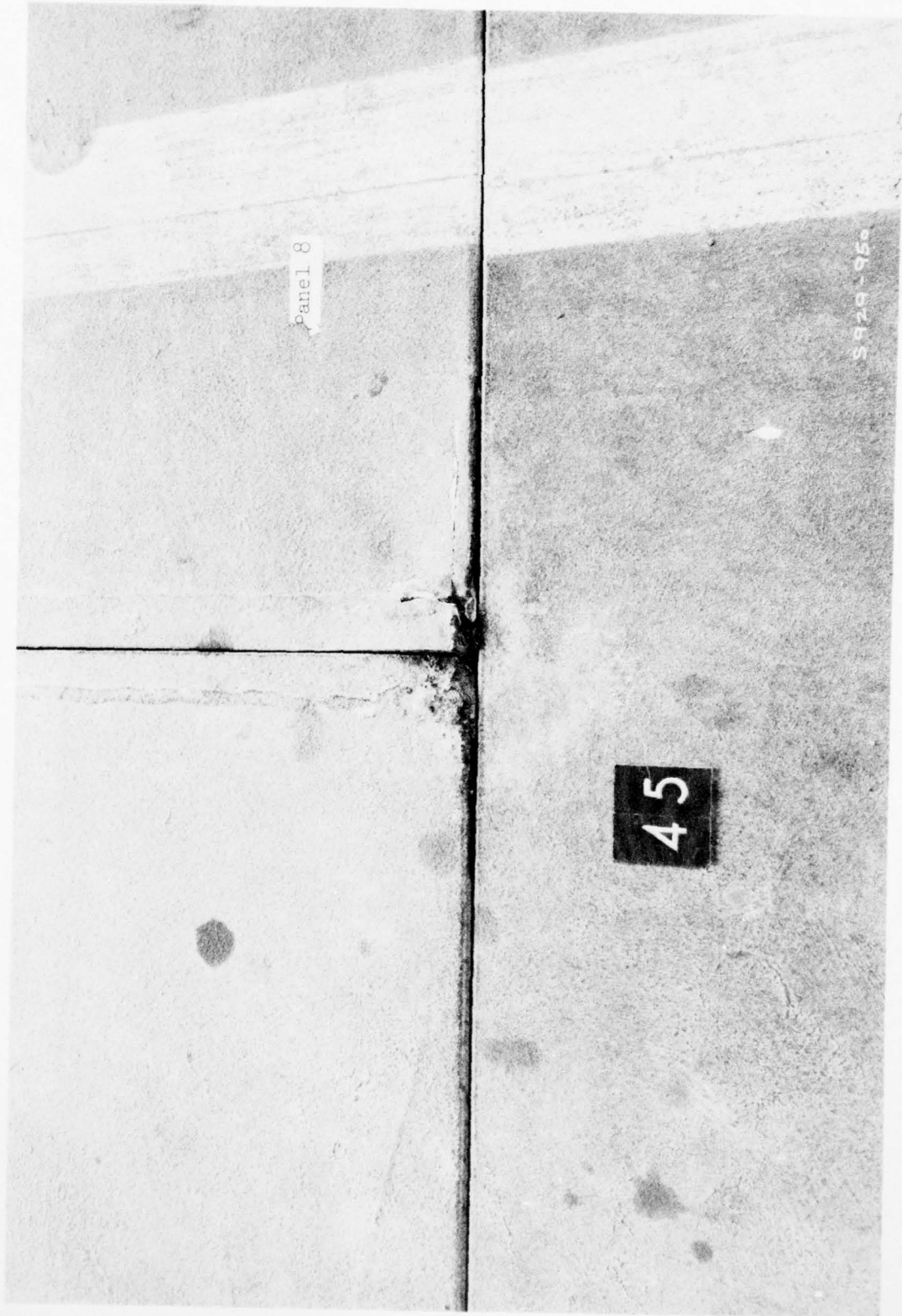
Crack in weld between I-lock and extrusion and split along male connector of panel 8 after 210 coverages, Phase 2, subgrade reprocessed
