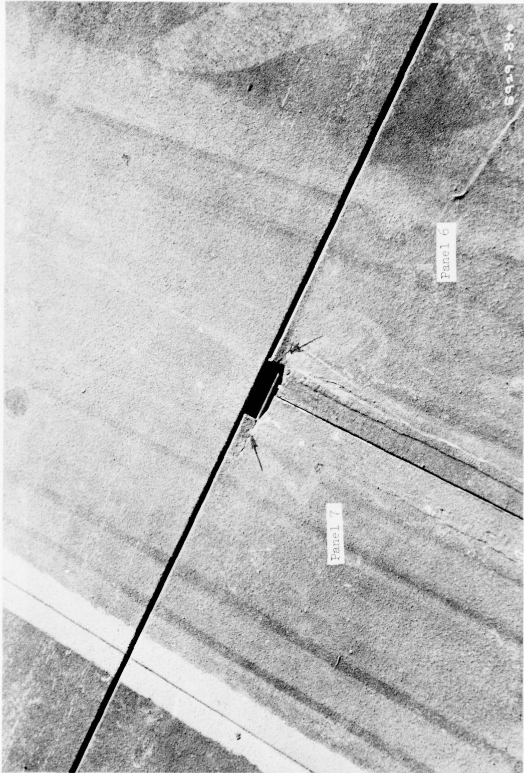
Curl on panels 6 and 7 (note antiskid flaking at corners)
