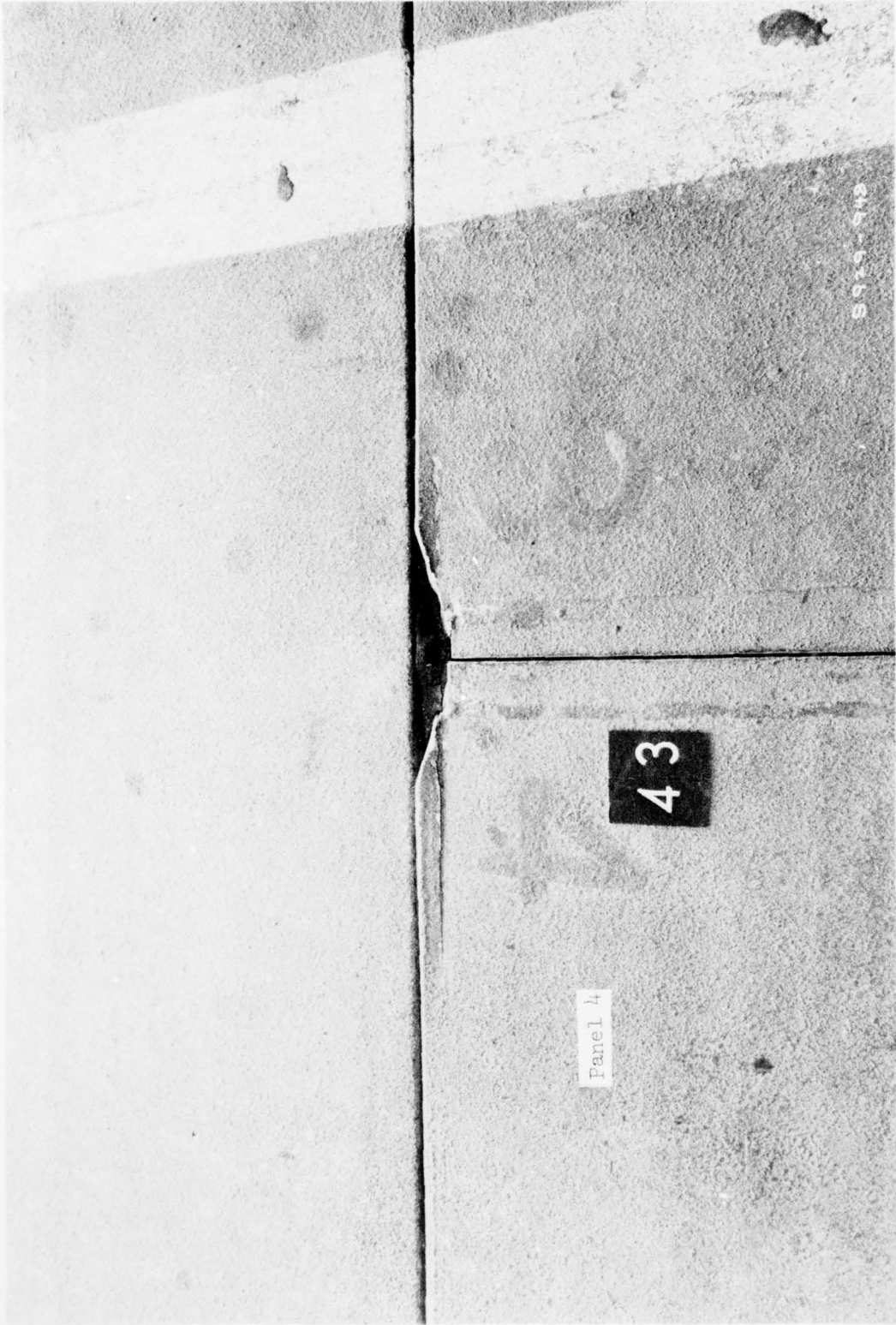
Split in female connector (west end) of panel 4 after 210 coverages, Phase 2, subgrade reprocessed
