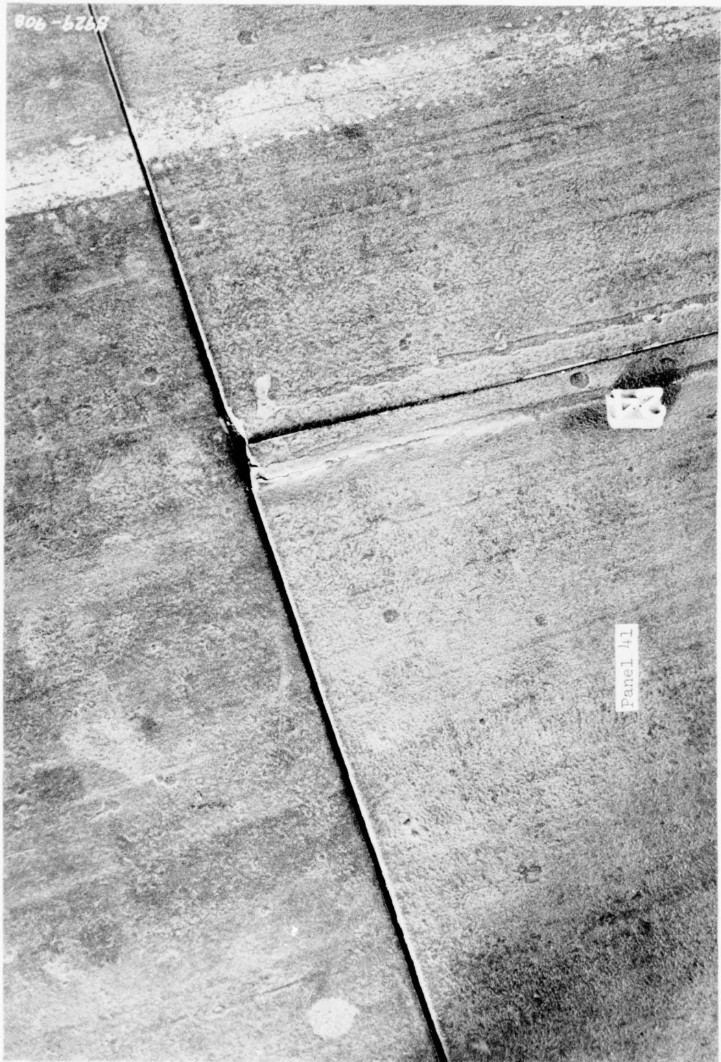
Weld crack at male I-lock corner of panel 41 after 1040 coverages, Phase 1
