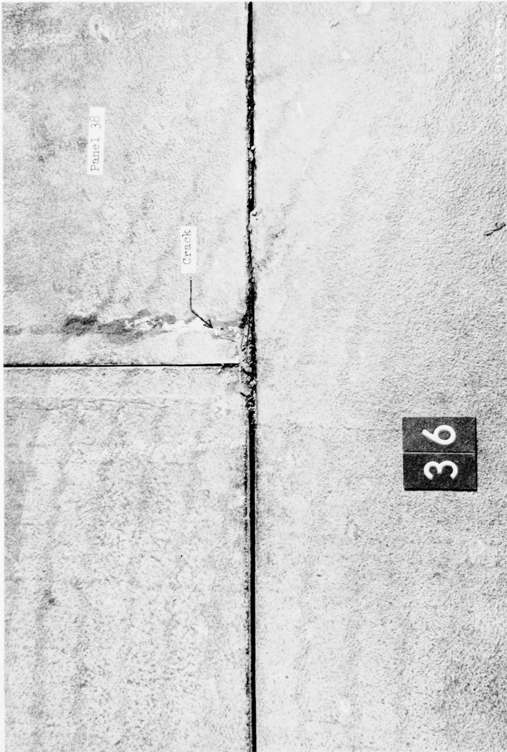
Crack in weld between I-lock connector and extrusion of panel 38 after 832 coverages, Phase 2
