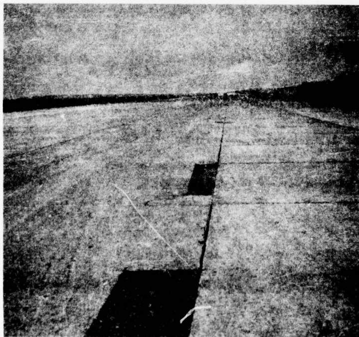
Photo 4. Patched joint spalls near north end of taxiway 26 (feature T4A)
