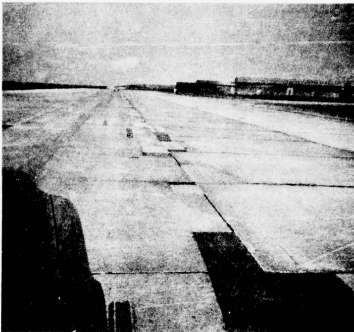
Photo 3. Patched joint spalls on taxiway 26 near parking apron. Note that patches are on each side of joint
