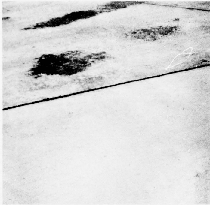
Photo 1. Scaling due to jet engine blast; south end of taxiway 5
