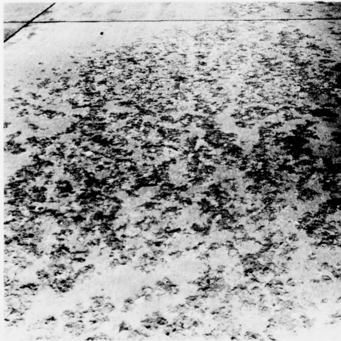
Photo 2. Fire-damaged slab in center wing parking apron
