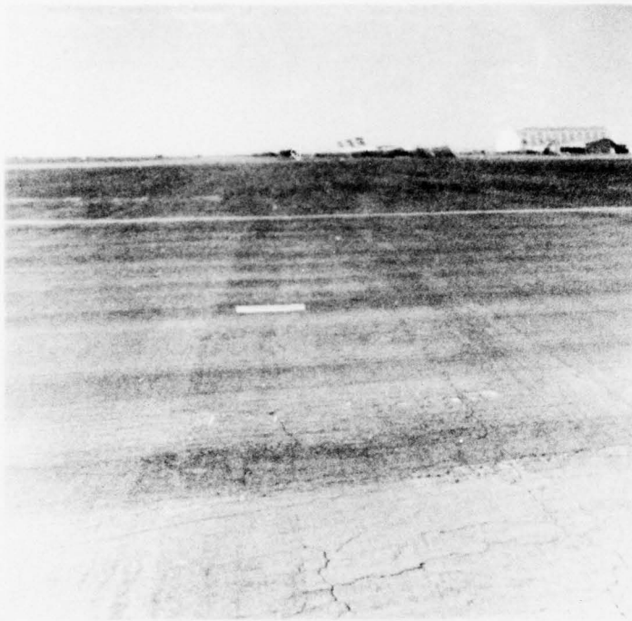
Photo 5. Cracking and rutting of AC pavement, south of taxiway 2 and adjacent to center wing parking apron
