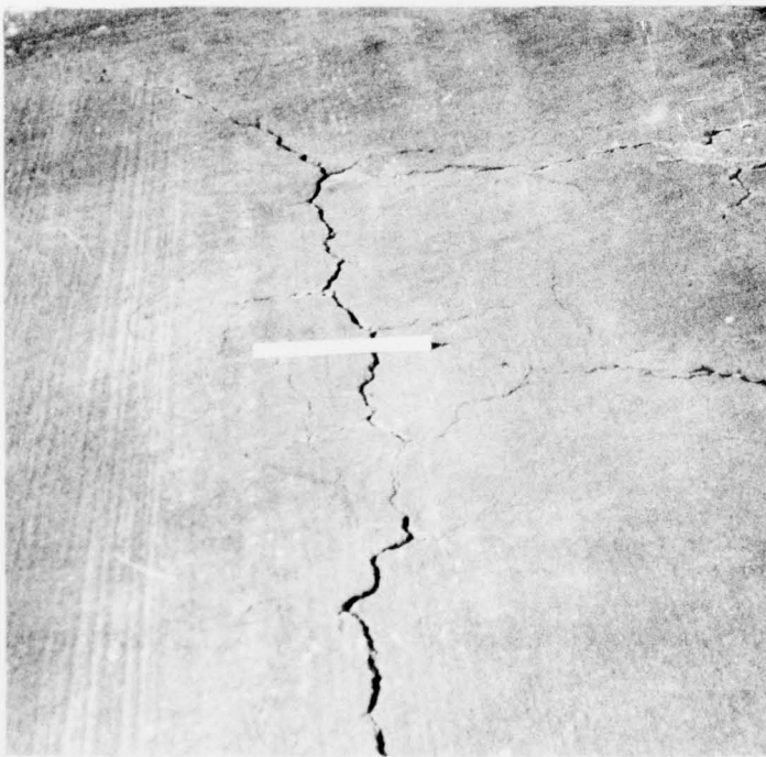
Photo 6. Cracking and rutting of AC pavement, south of taxiway 2 and adjacent to center wing parking apron
