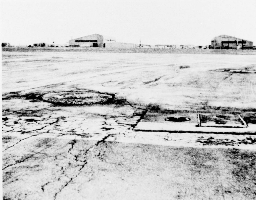
Photo 4. Taxiway R shoulder pavement. Note heaving adjacent to manhole on left
