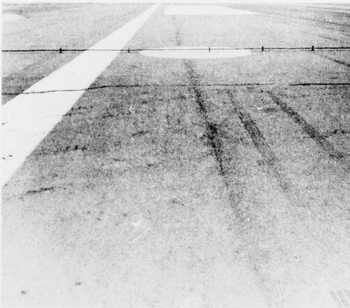
Photo 2. Longitudinal and transverse cracks near NE end of runway
