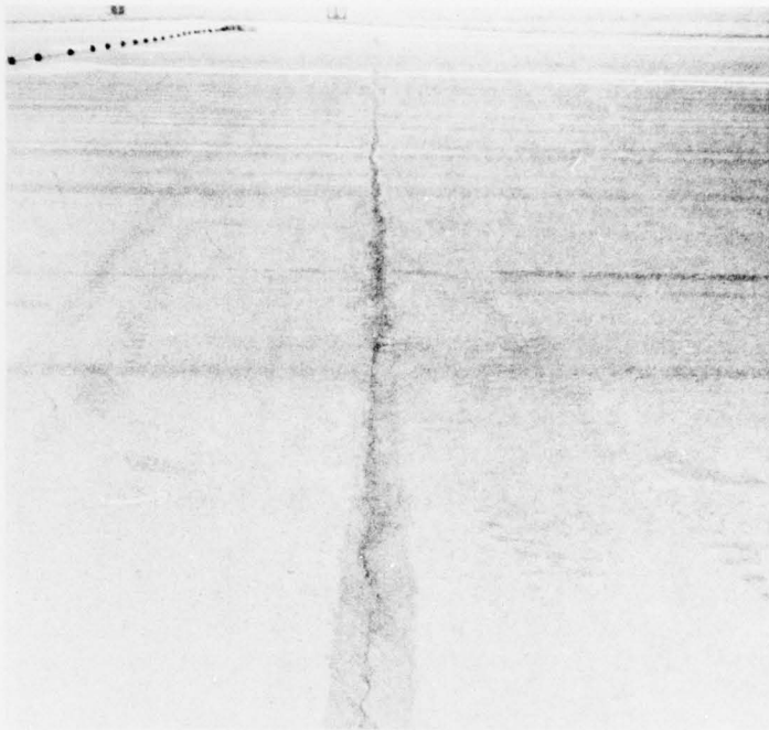
Photo 1. Transverse crack in runway near NE end
