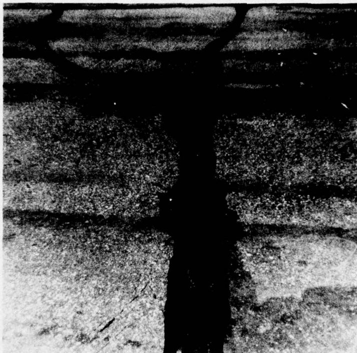
Photo 5. Cracks in taxiway B (feature T14B)
