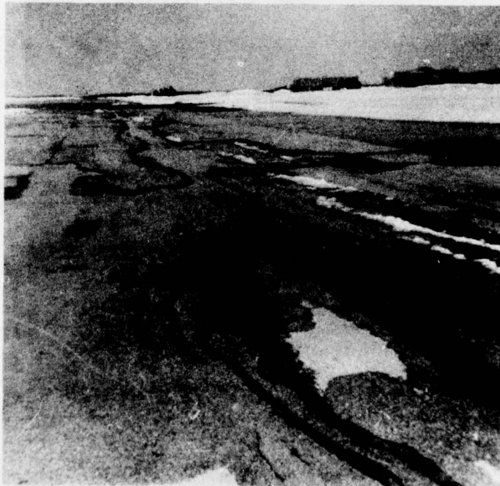
Photo 4. Rutting and longitudinal cracks in ADC alert access apron taxiway (feature T15B)
