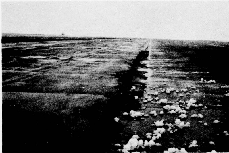
Photo 5. Shoulder pavement of parallel taxiway heaved 1-1/2 in. above edge of feature T11A
