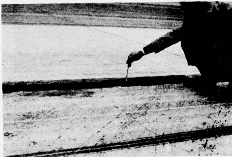
Photo 3. PCC runway keel heaved 2 in. above AC runway edge pavement near intersection of runway with taxiway C
