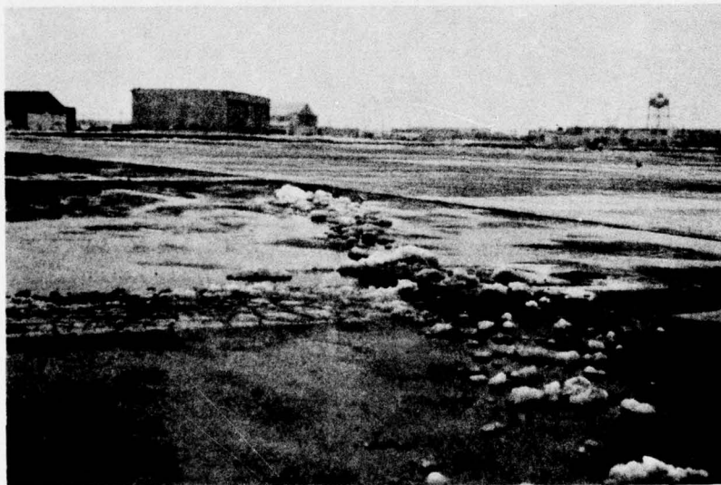
Photo 6. Differential frost heave at concrete insert in shoulder of taxiway B
