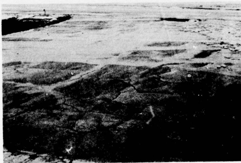
Photo 4. Random cracking of shoulder pavement at taxiway B caused by nonuniform frost heave
