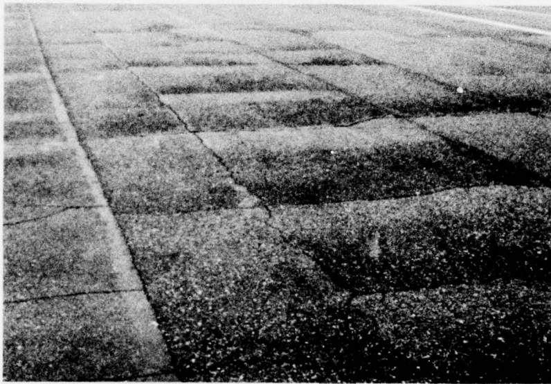
Photo 7. Transverse and longitudinal low-temperature contraction cracks at spacing of 10 to 15 ft in edge of primary taxiway (feature T11A)
