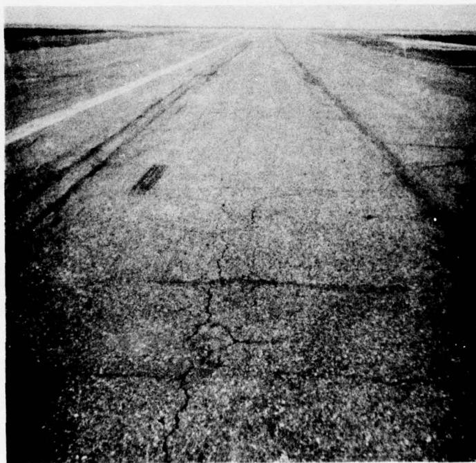
Photo 2. Random cracking in taxiway C
