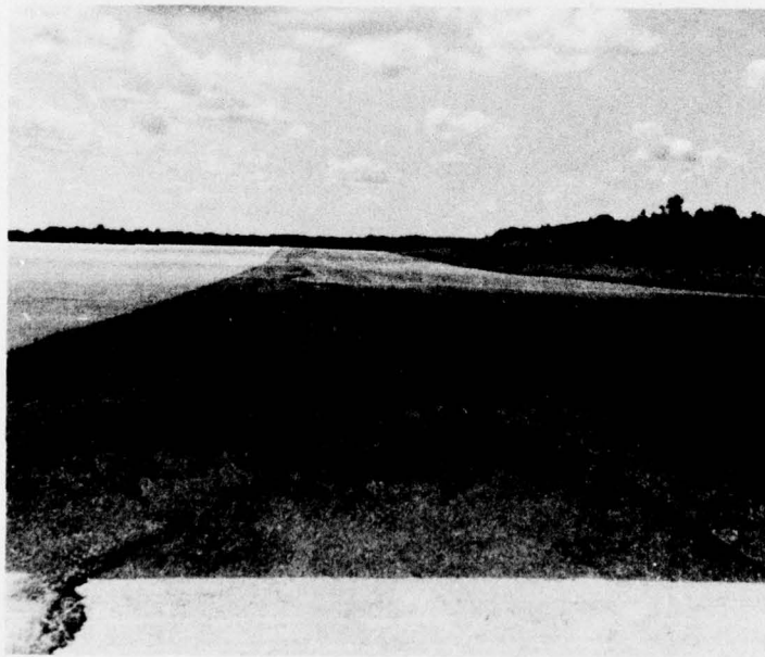
Photo 10. Upheaval of shoulder pavement at north end of parking apron A
