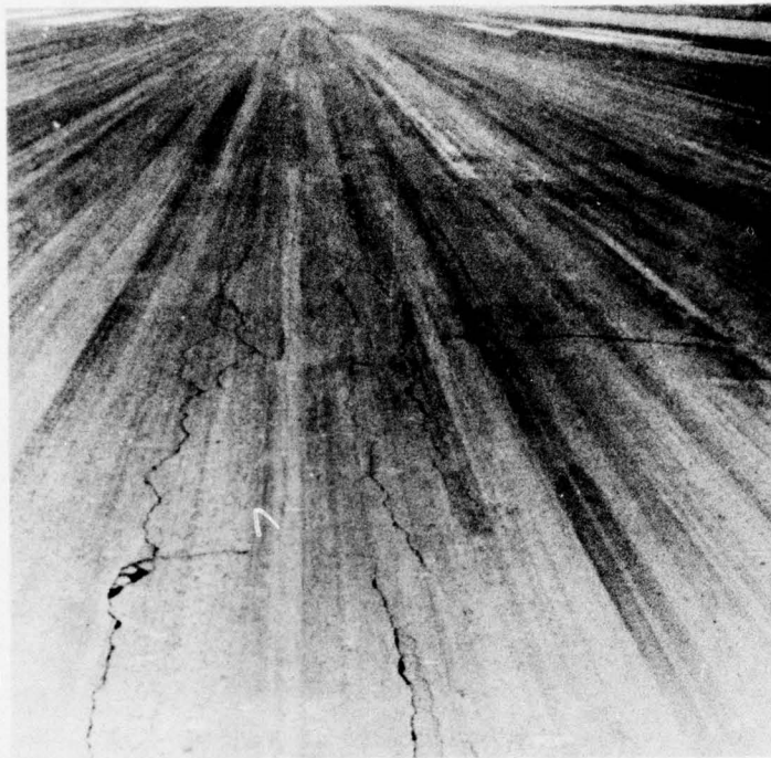
Photo 1. General view of cracking on runway approximately 2500 ft from NW end
