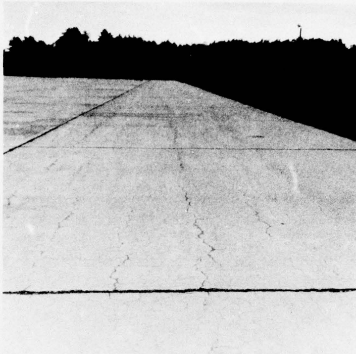
Photo 9. Typical longitudinal cracking (as in parking aprons A and B)
