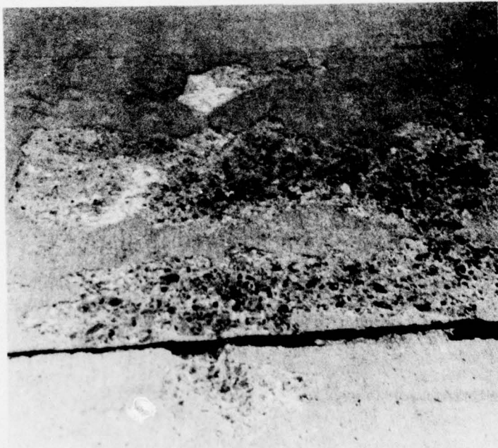
Photo 8. Scaling of slabs in south warm-up apron
