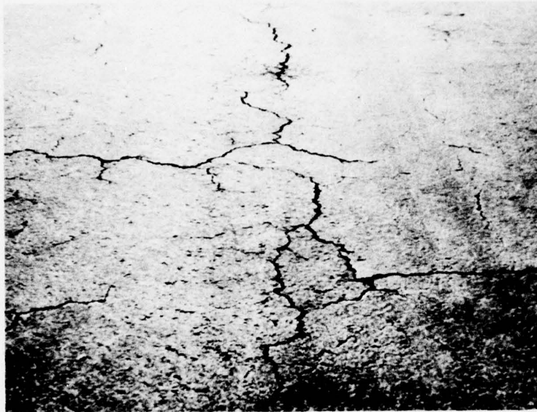
Photo 9. Typical poor condition of AC of transient apron
