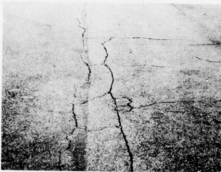
Photo 8. Typical cracks in AC pavement of refueling portion of parking apron
