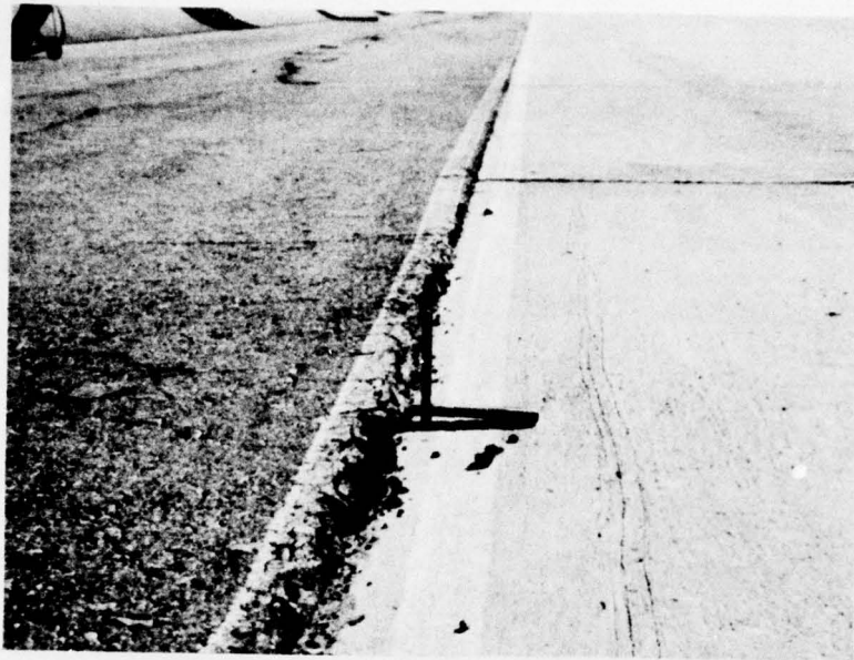
Photo 7. Upheaval of shoulder pavement along east side of parking apron near south end
