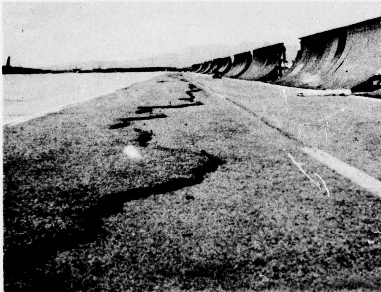
Photo 6. Showing of shoulder pavement along east side of parking apron near south end
