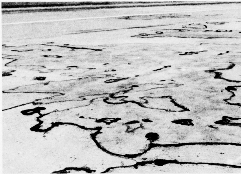
Photo 1. Epoxy patches near south end of runway
