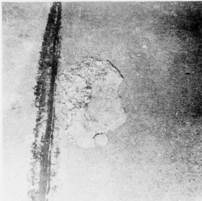
Photo 10. Scaling along joints from "D" cracking
