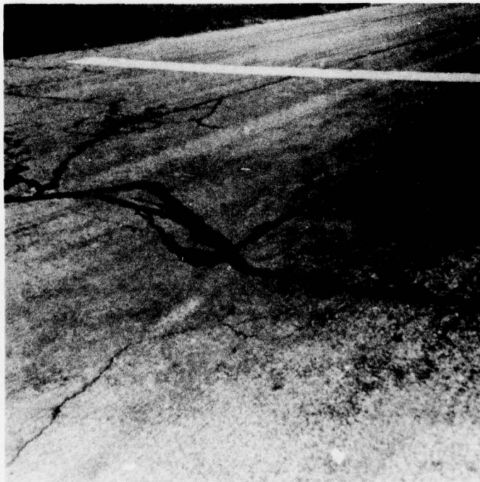
Photo 6. Condition of shoulder area adjacent to north warm-up apron
