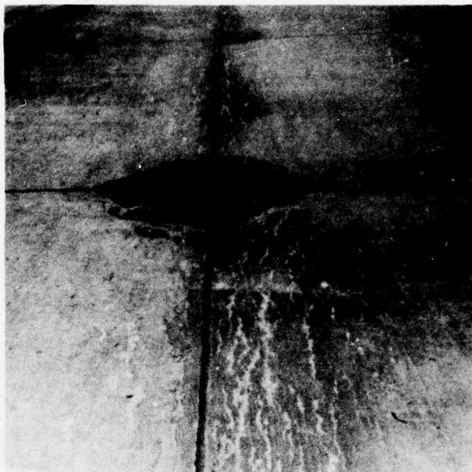
Photo 1. "D" cracking and corner spall repair on taxiway 16A
