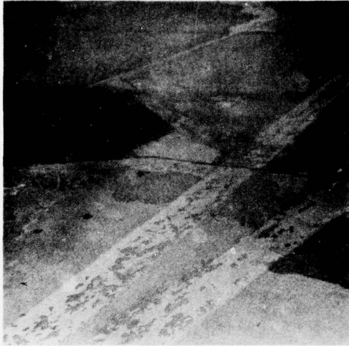
Photo 3. Water seepage through joints in apron
