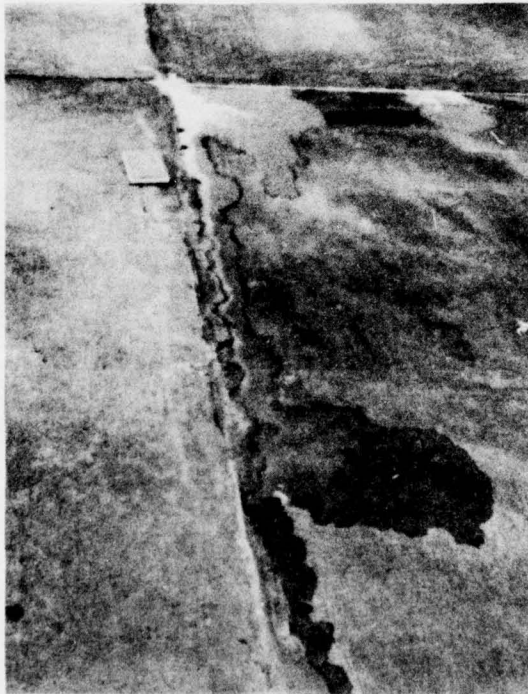
Photo 2. Water bleeding from joints in SE end of parking apron
