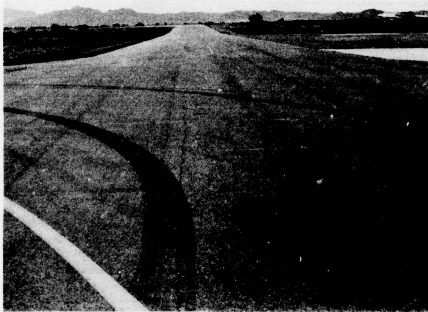
Photo 5. Surface condition of N-S taxiway (feature T3B). Overlay was placed in 1971
