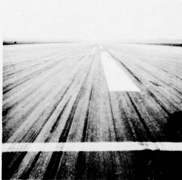
Photo 1. General view of AC overlay of runway interior (feature R3C) looking southwest from taxiway 15
