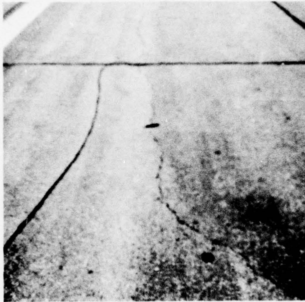
Photo 5. Reflection cracks in AC pavement of taxiway 1
