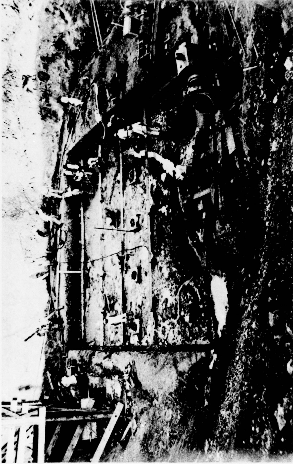
Photo 5. Carlson stress meters on foundation along east-west axis, prior to concrete placement
