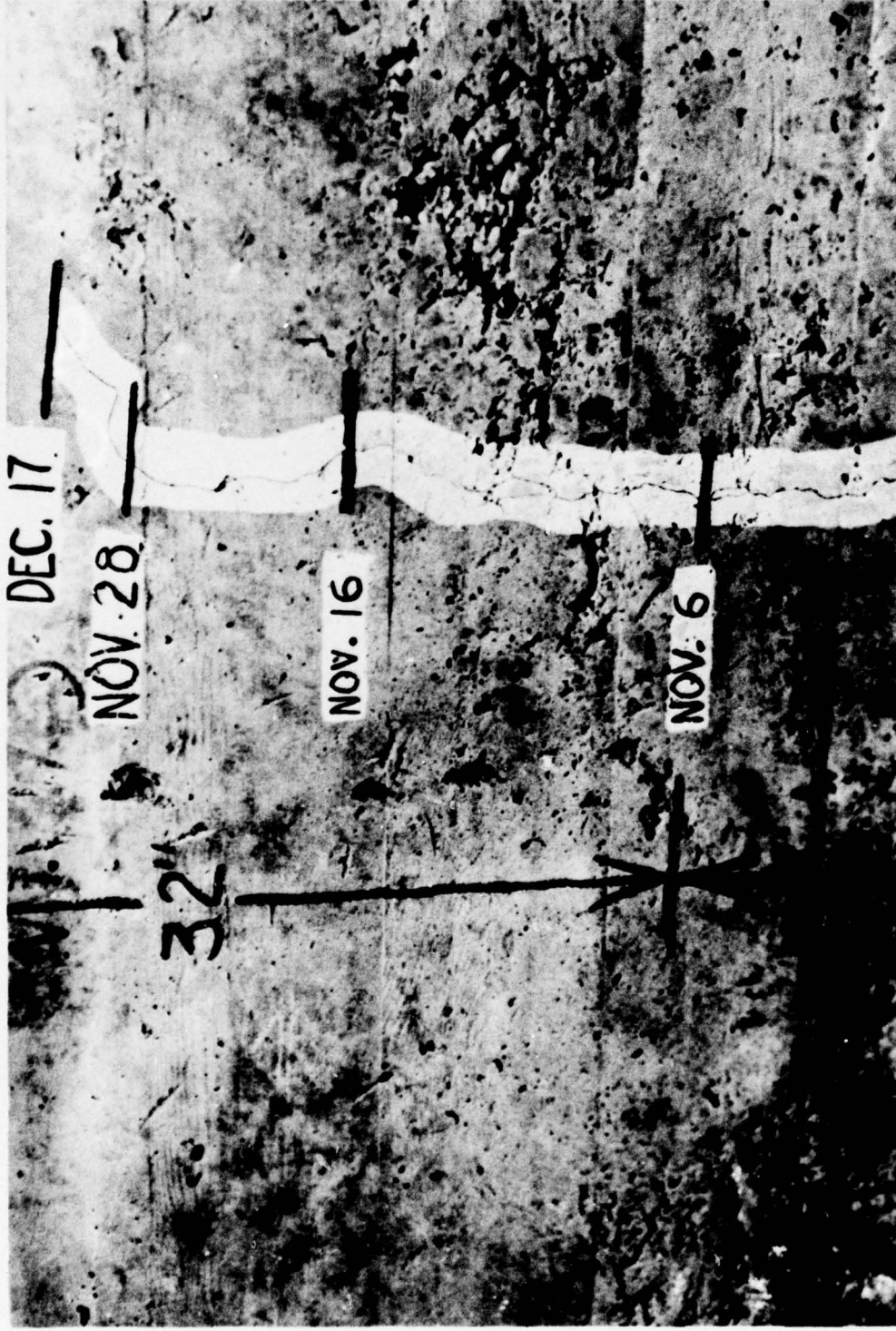
Photo 7. Crack on west side showing rate of development
