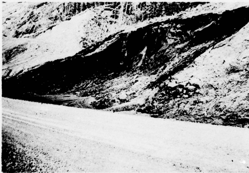
91. Close-up of start of sloughing, Mile 33.1 Rt, 26 June 1970.
