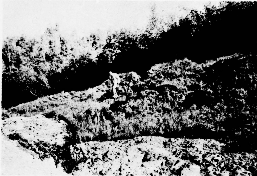
28. Most unstable portion of deep cut, Mile 9.85 Rt, 17 August 1971.
