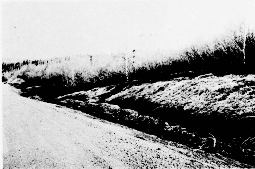
25. Relatively stabilized shallow cut, Mile 9.85 Rt, 28 May 1971.
