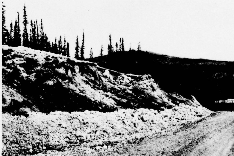
85. Gravel berm near base of backslope, Mile 23.2 Lf, 28 May 1971.
