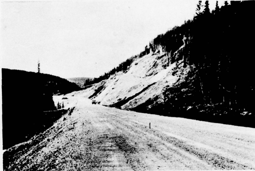
90. Overall view of backslopes, Mile 33.1 Rt in foreground and Mile 33.3 Rt in background, 26 June 1970.
