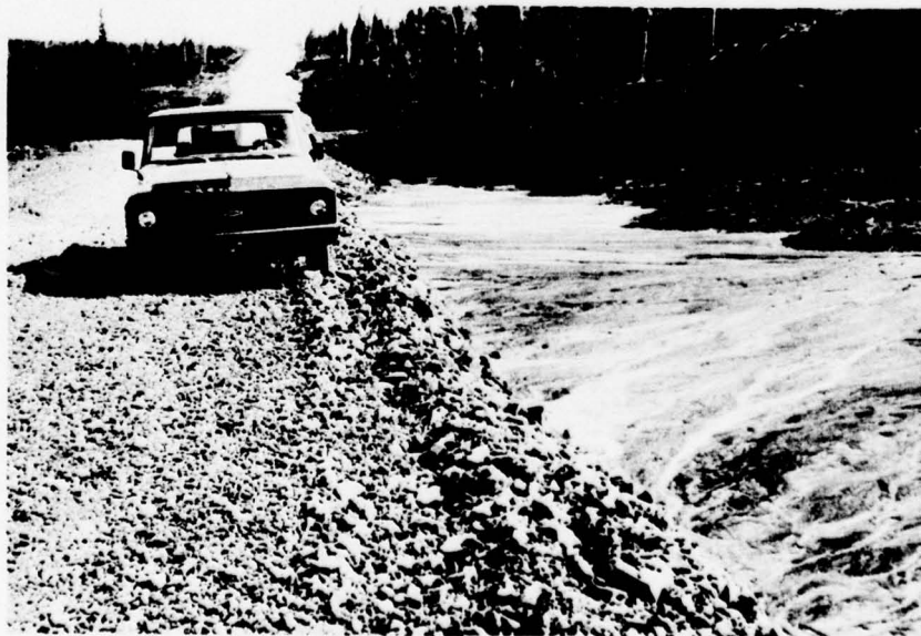
33. Backslope erosion into parallel ditch, Mile 19.6 Lf, 26 June 1970.
