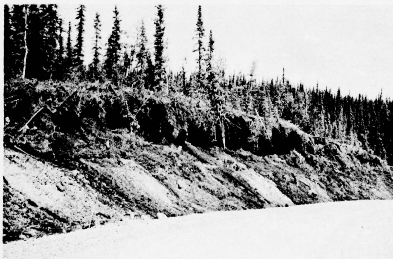
57. Ice face with overhanging mat and hydroseeded lower portion of slope, Mile 20.25 Lf, 11 August 1970.
