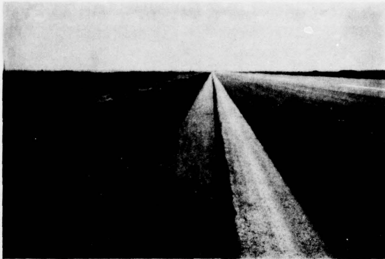
Photo 3. Edge of primary runway indicating area that had not received hot-mix plant seal in 1973
