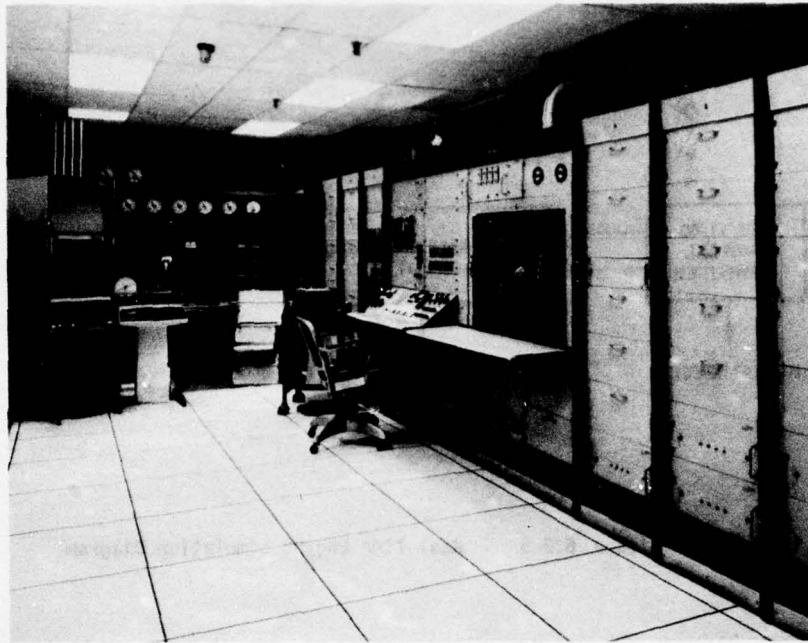
Figure 6.2-3 CLB Control Room
