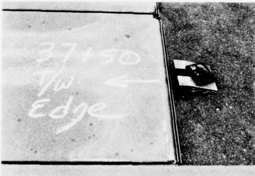
b. Radius mat shifted west away from anchor Taxiway shifting at 300 sorties
