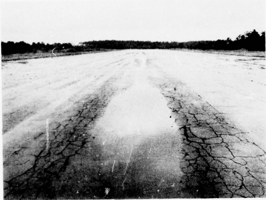
Deteriorating asphalt on runway 27-90
