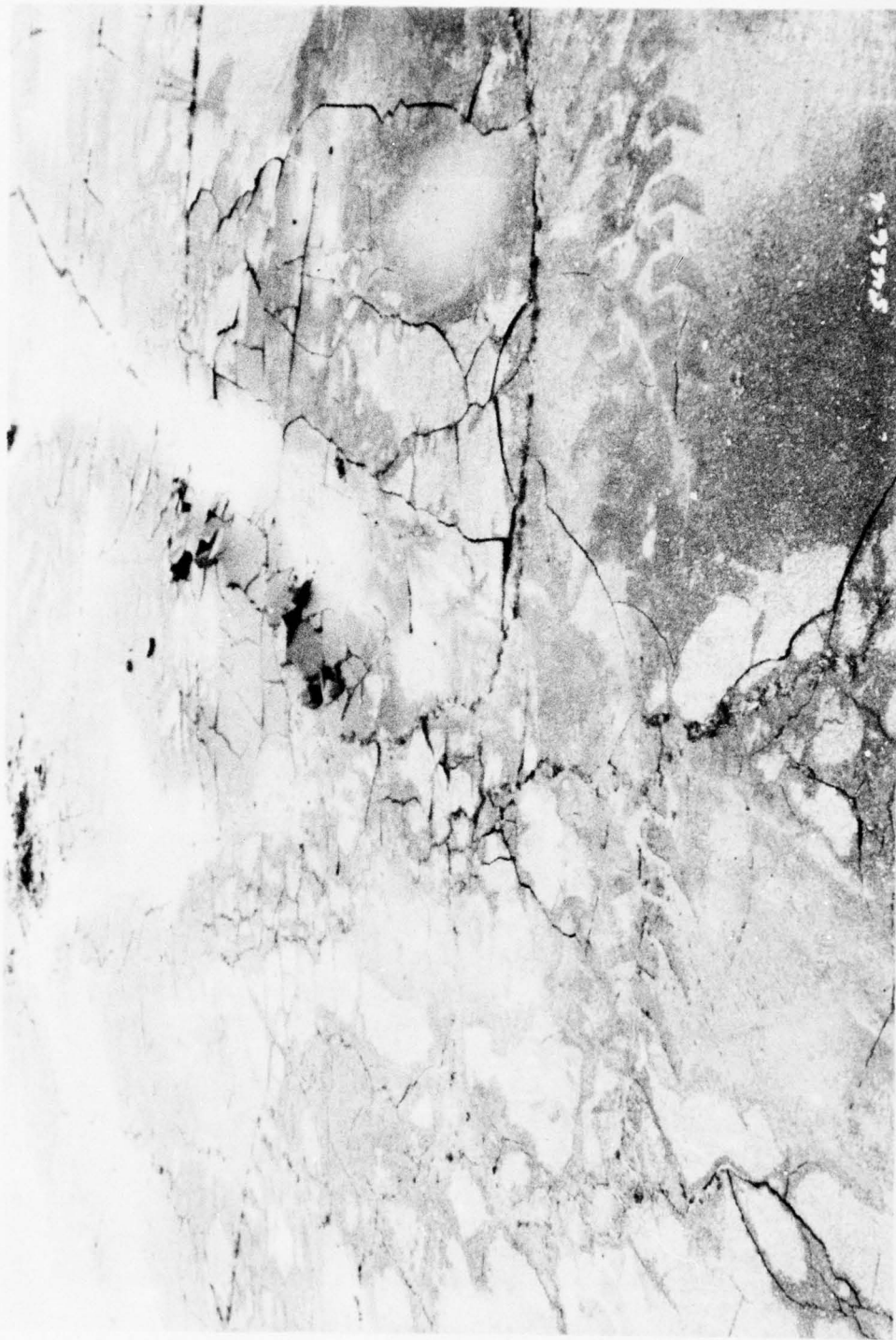
Rutted and broken asphalt in overrun area on south end of runway 18-36
