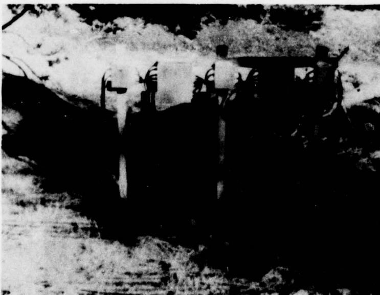
Figure 50. A typical multiple cable trail junction box installation
