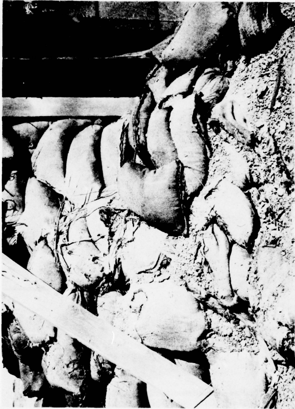
Fig 17 Sandbag and mount support damage, Test No. 2
