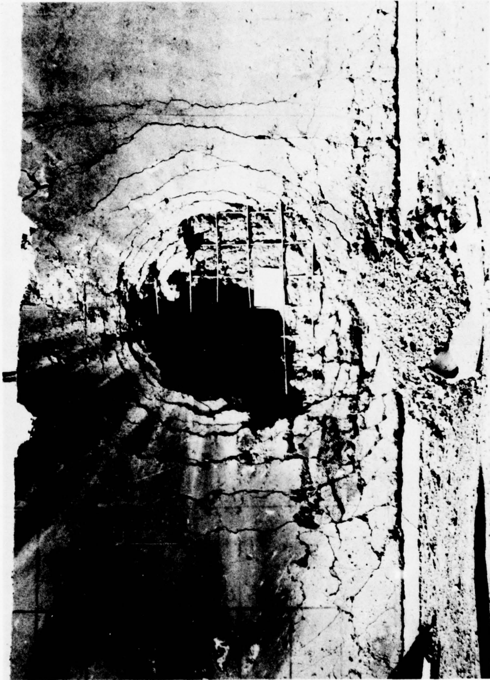
Fig 19 Front face damage, Wall No. 1, Test No. 3
