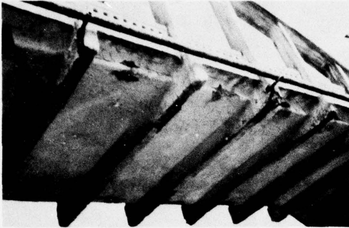
a. Overall view. (The utility line is anchored to the floor beams)
