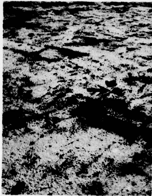
Figure 1. Daytime photograph of a portion of the northerly roof, Building 33. The arrow points to the location of sample A.
