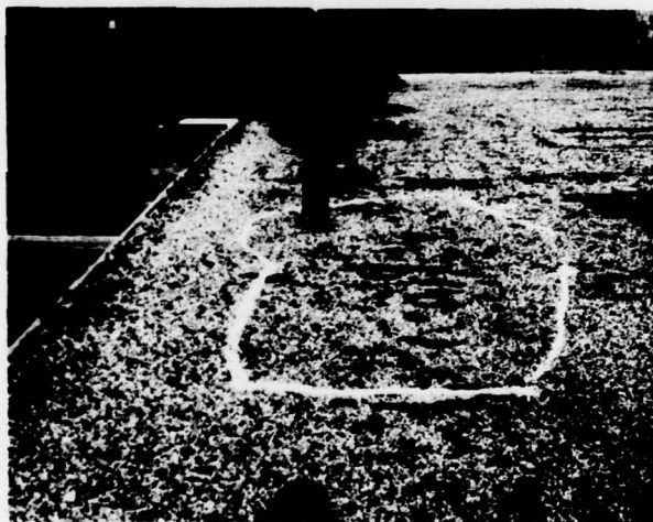
Figure 9. Area in bay 1, Building 122, that showed up bright in the infrared camera. Its boundary was marked with spray paint.
