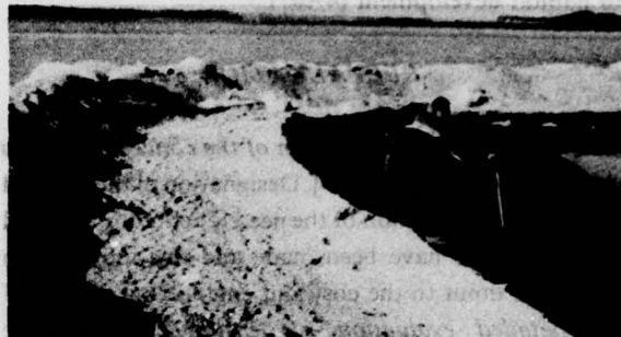
Figure 7. A portion of a 1000-m dike used in marsh development in the James River, Virginia. The dike, built from sandy dredged material, provides containment for fine-textured dredged material and protection for a freshwater marsh established at this high-energy riverine site
