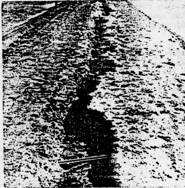
Figure 5-19. Crack along the crest of a dam on the Yukon River.
