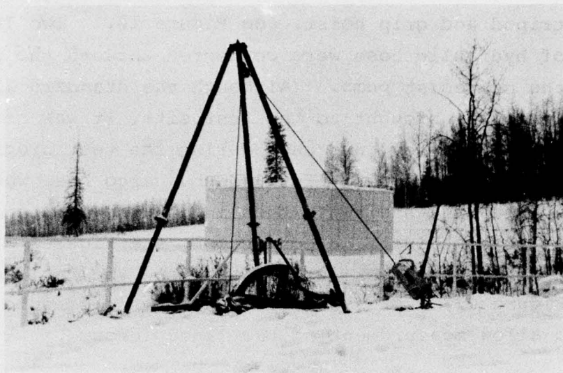
Figure #18: Tripod, Grip Hoist, and Hose Saddle on Storage Tank Top
