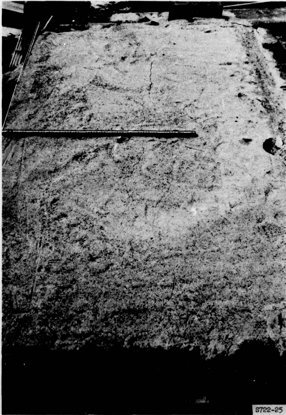
Figure 28. Development of surface cracks two months after the construction of the wall
