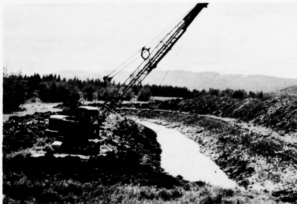
Constructing irrigation pond with dragline to make underground water readily accessible. (SCS F-134-4)
