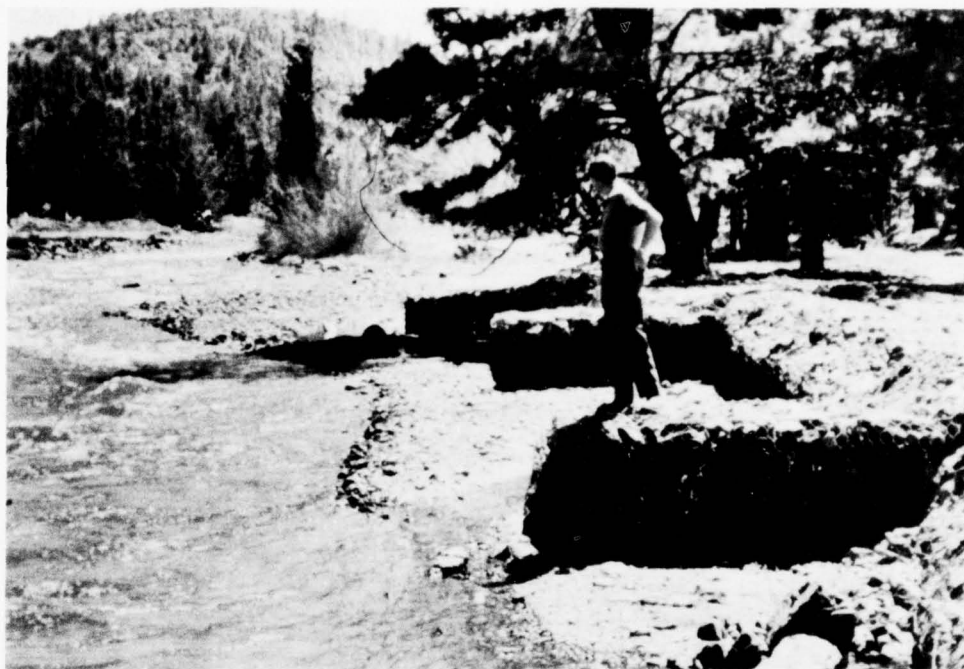
Streambank protection work along the Chequamegon River. This type of revetment, large-sized gravel contained in wire baskets, holds many cubic yards of loose streamside soil in place. (Forest Service)
