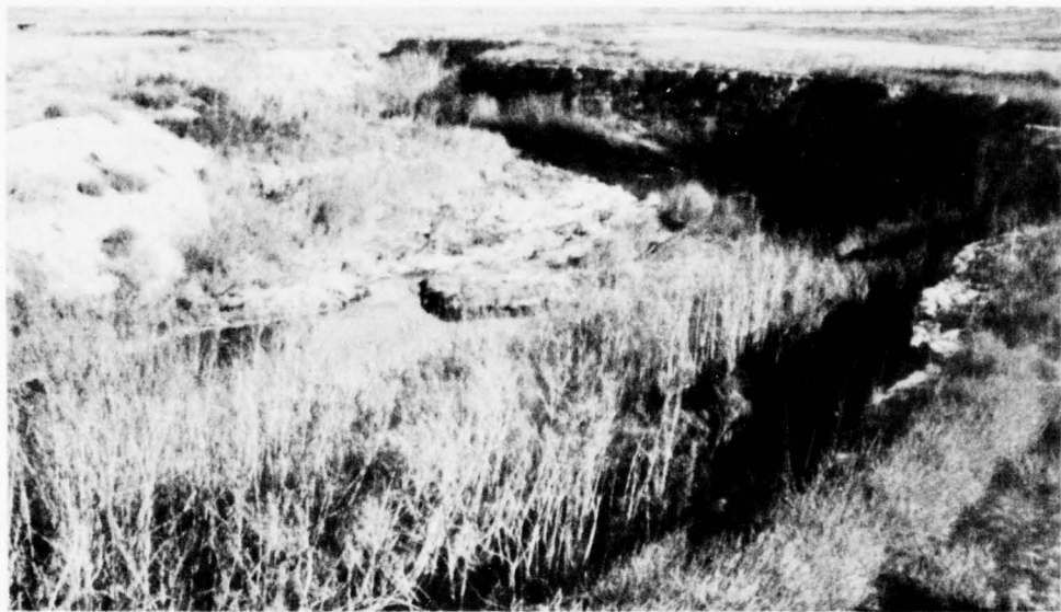
Bank erosion gradually destroys the most productive soils. Land destroyed and soils lost in this way cannot be reclaimed. Sediments from these areas can damage down stream areas. (SCS 0-994-7)
