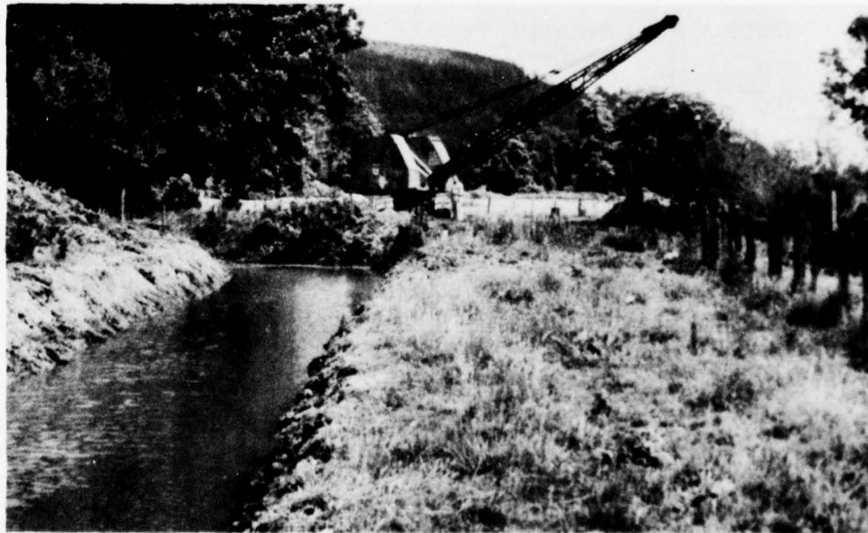
Open drainage canals and laterals are common practices for removing excess water in this subregion. (SCS F-99-12)
