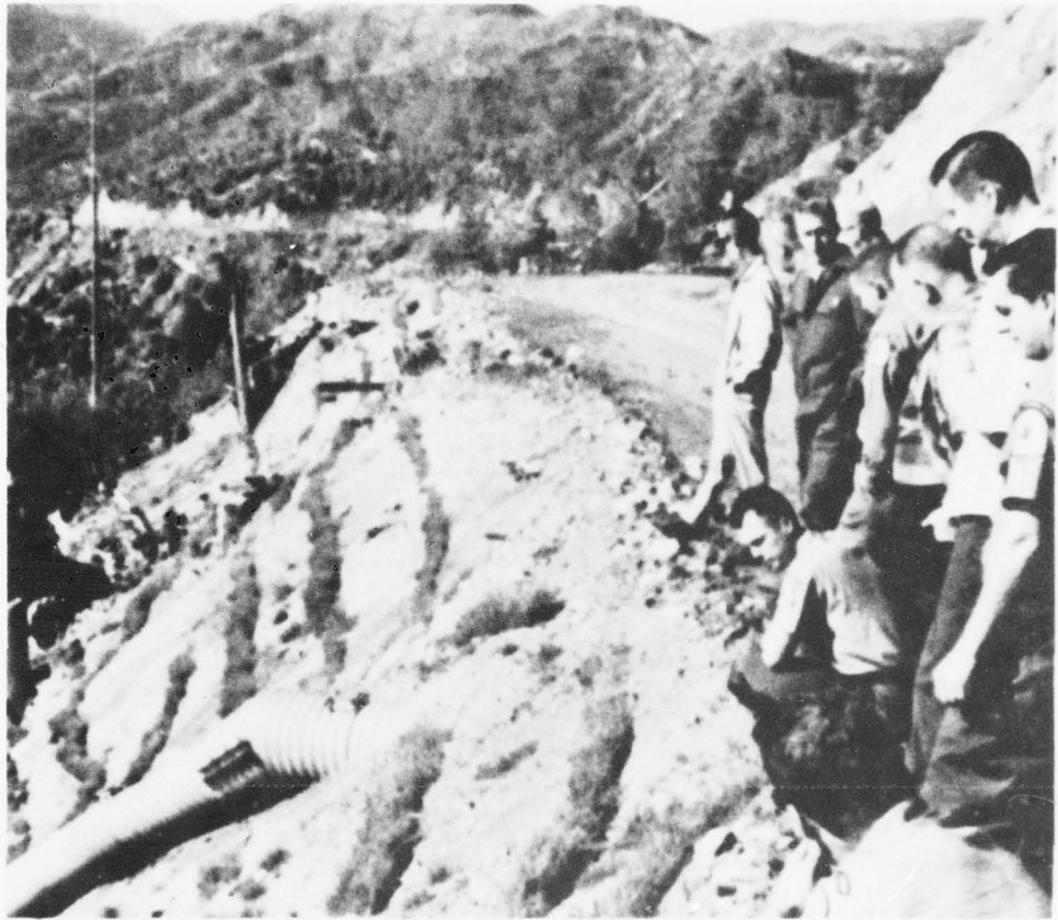
Seeding in furrows, an attempt to retain soil moisture and reduce gullying on steep fill slopes. (Forest Service)
