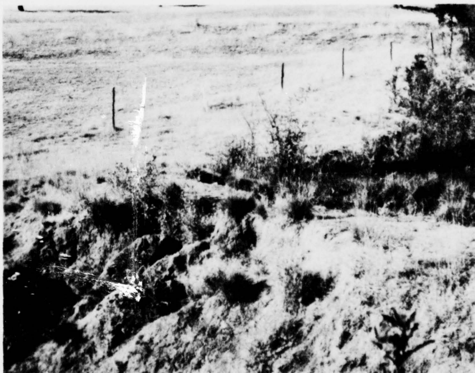
Erosion occurring on a dam of a small stock water pond is due to lack of maintenance and on improperly constructed spillway. A number of water facilities are needed in this subregion and many will require reconstruction or maintenance work. (SCS 0-2198-18)
