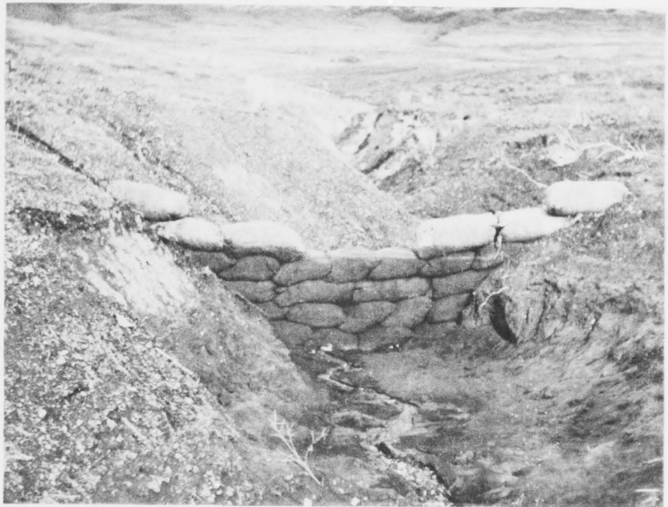
Check dams help retard excessive runoff and silt deposits, by channel stabilization. Other measures are needed to reestablish desirable plant cover on the watershed. (Bureau of Land Management)
