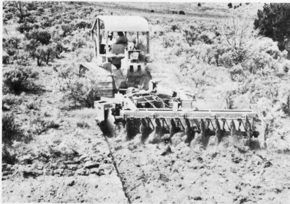
Range areas are plowed to kill undesirable species that do not give adequate ground cover. This practice prepares a seedbed for vegetation which is more useful, protective, and erosion resistant. (Bureau of Land Management)
