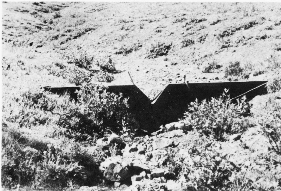
A number of check dams have been constructed to prevent channel cutting while protective vegetative cover is being re-established on eroding slopes. Note sediment deposit being held behind this structure. (Forest Service)
