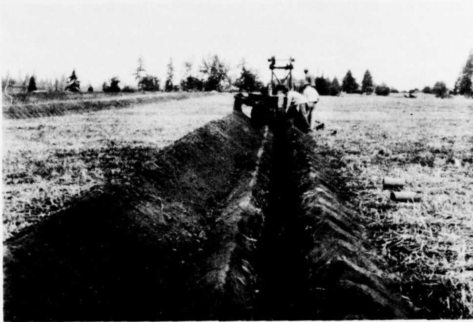
Subsurface drainage can be accomplished by properly designed and installed tile systems. (SCS 7-1049-7)
