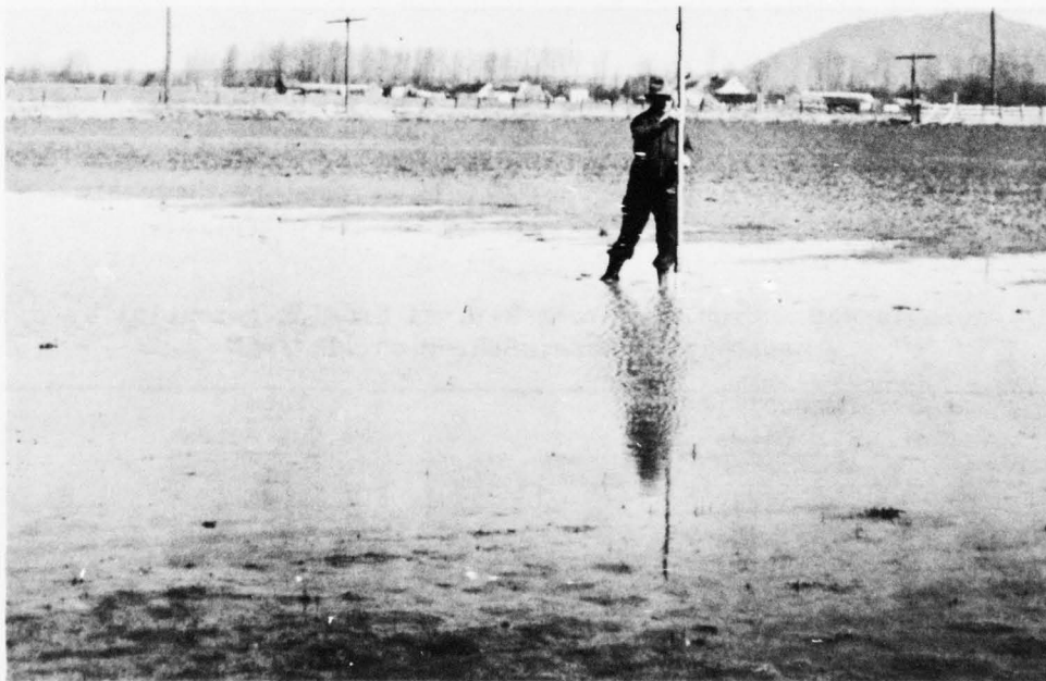
Surveying for the installation of a tile drain to remove excess surface water and to drain the soil profile. (SCS W-1145-7)
