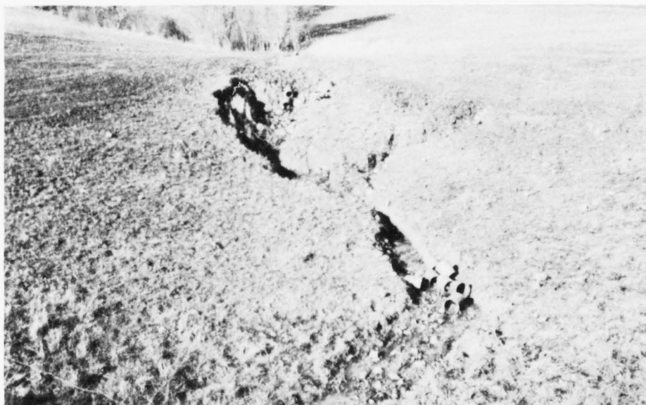
Poorly designed tile drain system failed to function properly causing gullying and did not serve the function for which it was intended. (SCS 7-538-9)
