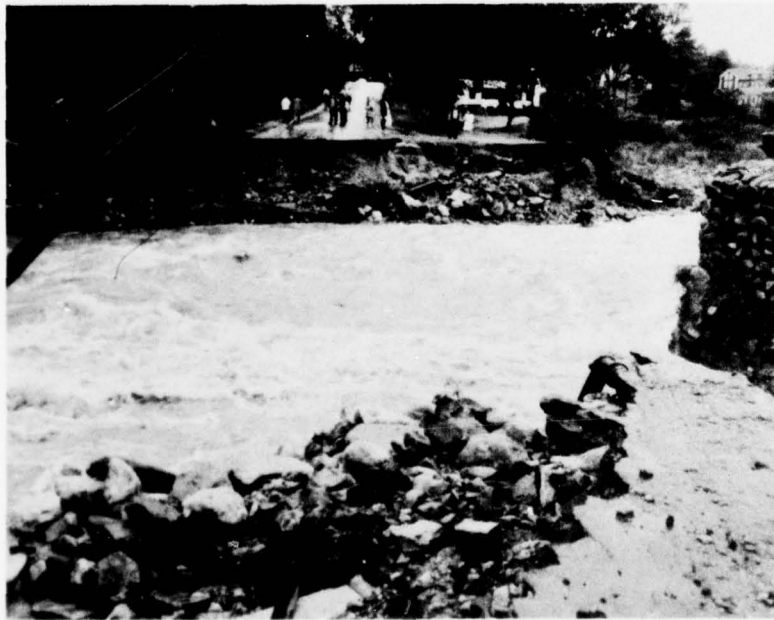
Rampaging stream waters have washed out bridge. Necessity of rerouting traffic is an indirect damage.
