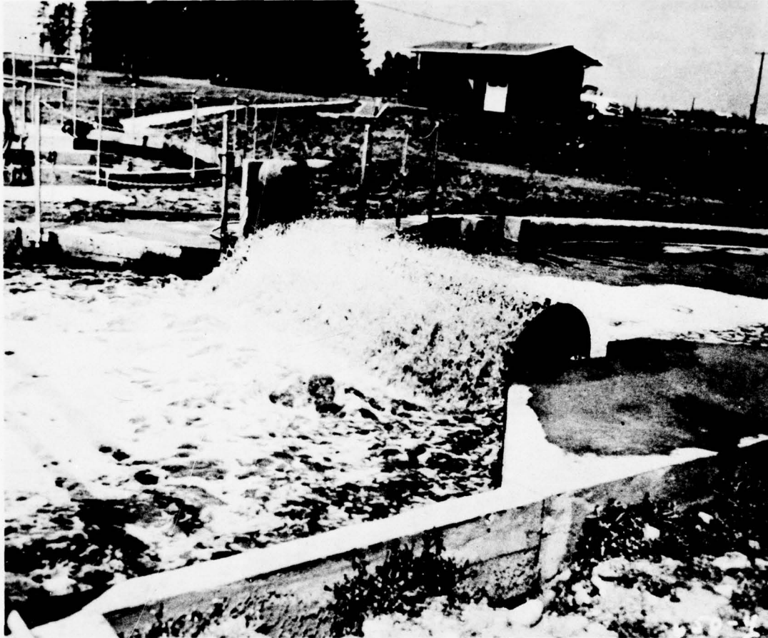
Photo IV-6. One of the mechanical aerators in operation at the Stayton treatment plant. (Department of Environmental Quality, Portland, Oregon, Photo)
