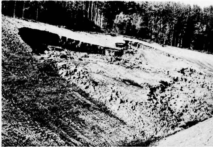
Plate 33. Pump Station 11: Massive deep seated slope failure. Failure began about mid-June after a period of heavy rainfall. Some additional sliding occurred about mid-July. Seeded latter part of June.
