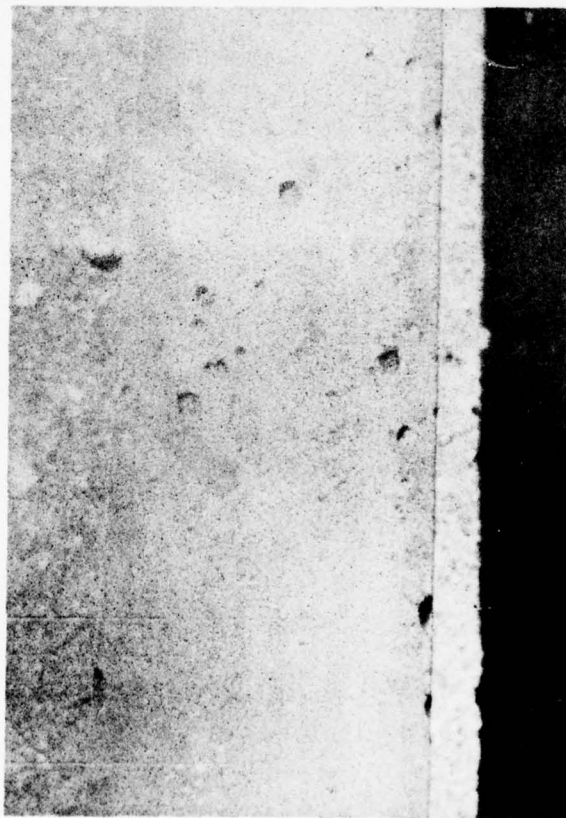
Figure A9. Aluminum-pigmented epoxy tar after sandblasting. Pitting is evidence of damage in the immersed zone.
