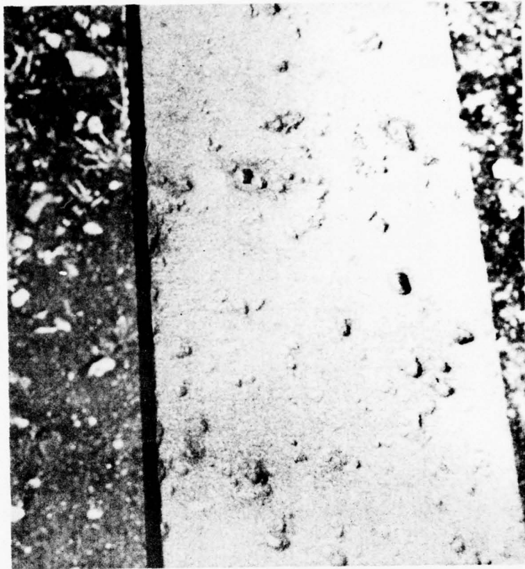
Figure A10. Epoxy-tar over zinc-rich primer after sandblasting. Severe pitting in the immersed zone is indication of structural degradation caused by corrosion.
