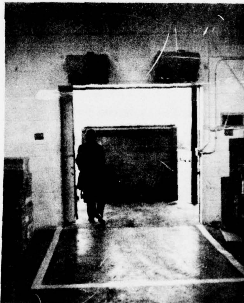
c. Same problem as b. Note damage to unit on right.
