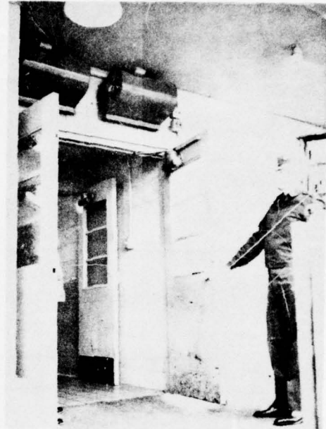
b. Air curtain machine does not provide continuous full-width coverage at top of door.
