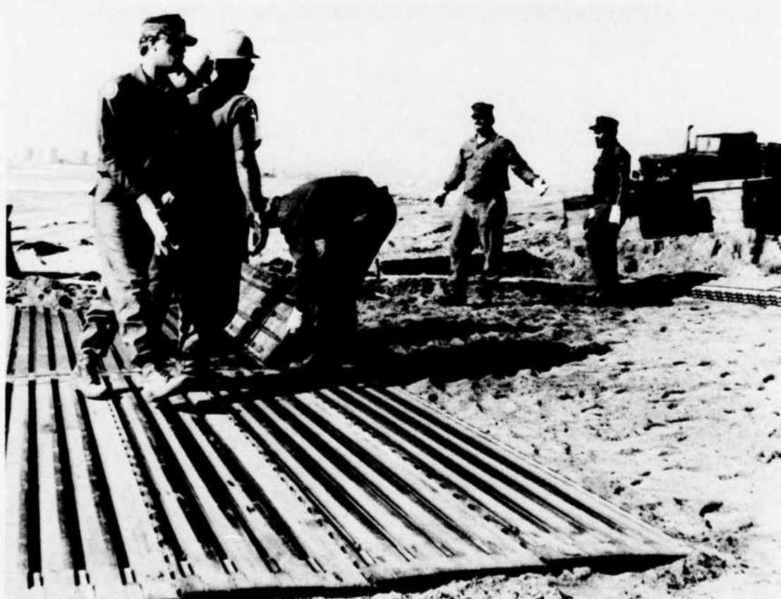
Figure 10. Steel mat, M8A1, used to support container crane and container transporters across beach.
