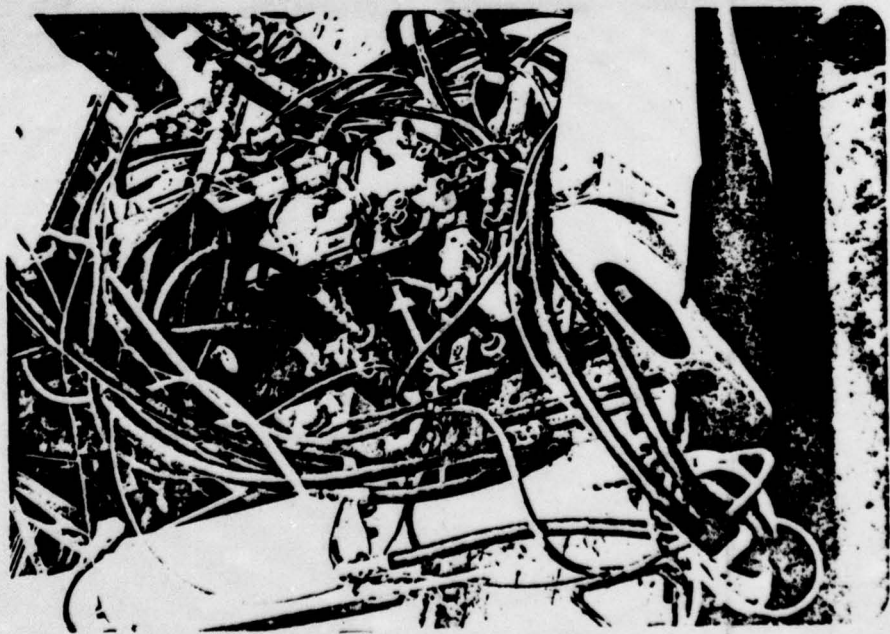
Figure 16. Photographs of the HP system.
