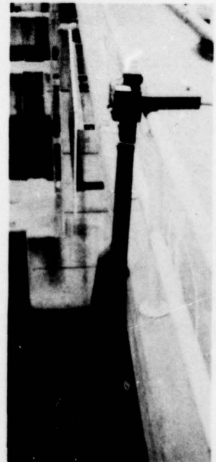
Figure 9. Optical flowmeter mounted on spillway bridge above spillway bay 8
